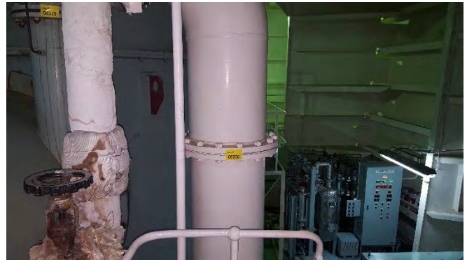
Photo 46 G6206 3rd Deck - IGG Room, Burner Outlet Manifold – Gasket (UMF)
