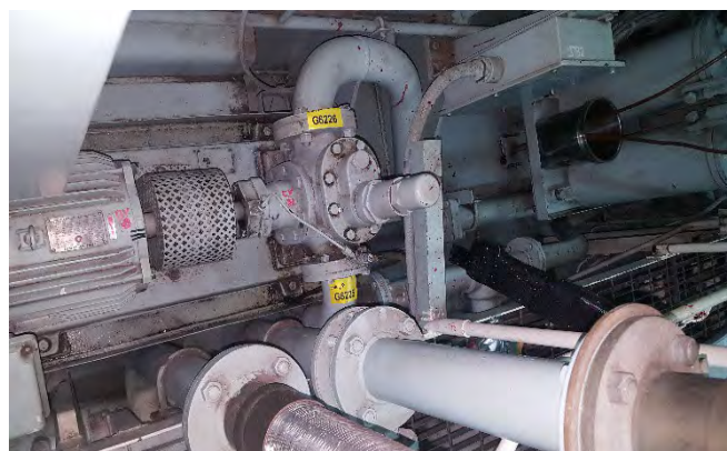
Photo 54 G6226 3rd Deck - No.2 Diesel Alternator Room , Lube Oil Pump Suction, Flange – Gasket (Chrysotile)
