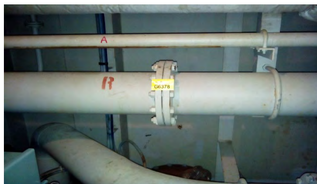
Photo 114 G6378 Upper Deck - Pipe Passage Starboard, .HFO Bunker Pipe Flange (Aft) – Gasket (UMF)
