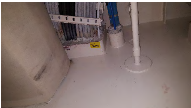
Photo 139 G6318 F Deck - Electrical Cable Trunk Room, Starboard, Cables Through Bulk Head - Bulkhead penetration insulation (Chrysotile)
