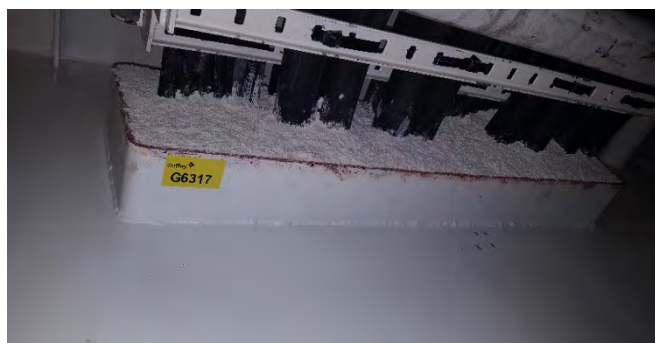
Photo 138 G6317 F Deck - Electrical Cable Trunk Room, Starboard, Cables Through Bulk Head - Bulkhead penetration insulation (Presumed Positive) (Chrysotile)
