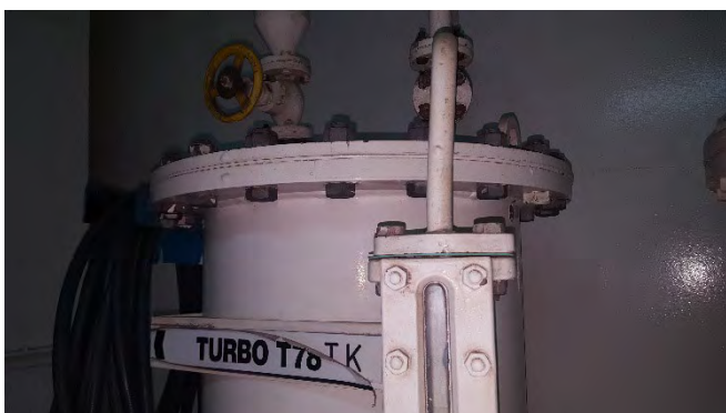
Photo 65 Refer to G6289 3rd Deck Engine Room, Turbo T78, Lube Oil Gravity Tank Level Sight Glass Flange - Gasket (Chrysotile)
