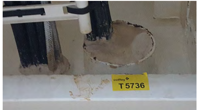
Photo 32 G6143 3rd Deck - Workshop Mezzanine, Port, Aft, Small Penetration for Electrical Conduit – Bulkhead penetration insulation (Off-White in colour) (Chrysotile)
