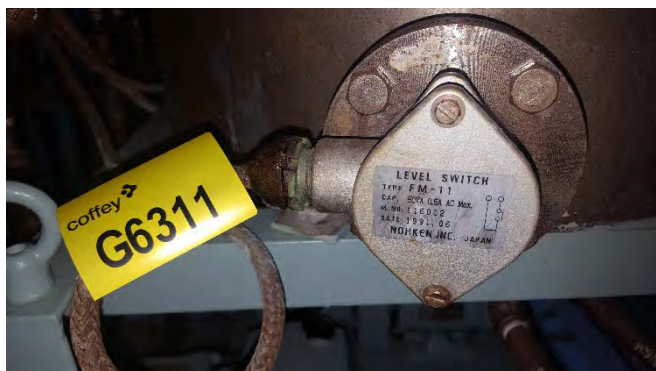
Photo 93 G6311 2nd Deck Chemical Locker, Boiler, Chemical Dosing Tank, Low Level Switch – Putty (Soft) (Presumed Positive)
