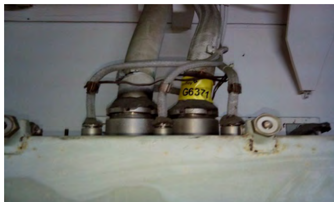
Photo 110 G6371 Upper Deck Forecastle/Bosun Store, No.2 Winch and Windlass Hydraulic Pump Power Cabinet Connection – Putty (Chrysotile)
