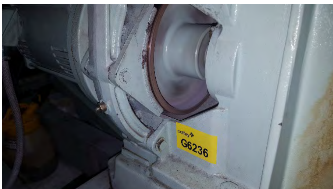
Photo 57 G6236 3rd Deck Lift Motor Room, Brake System Friction Material – Lining (Chrysotile)
