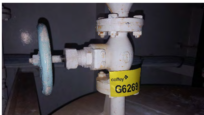
Photo 95 G6269 Upper Deck Forced Draft Fan Flat, Cooling Water Header Tank Filling Valve - Gasket (UMF)
