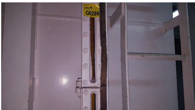
Photo 63 G6289 3rd Deck Engine Room, Turbine, Lube Oil Gravity Tank Level Sight Glass Flange – Gasket (UMF)
