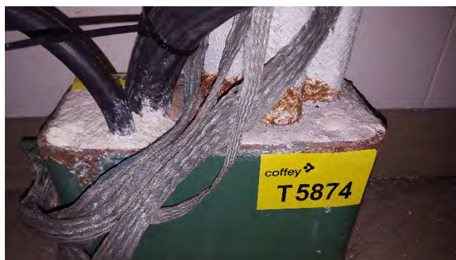
Photo 136 T5874 F Deck - No.2 Equipment Room, Bulkhead penetration insulation (White/Hard) (Presumed Positive) (Chrysotile)
