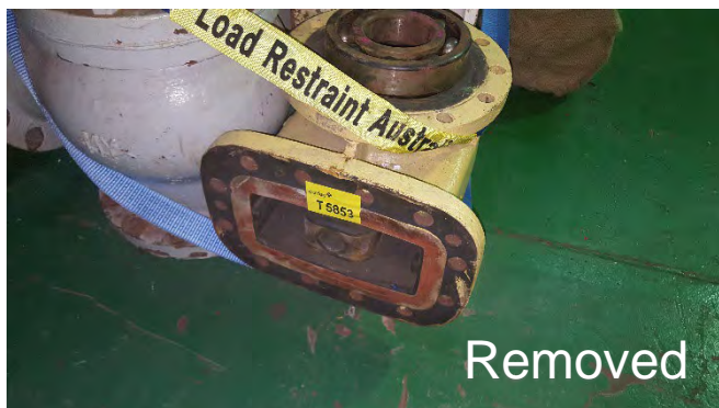
Photo 79 T5853 2nd Deck - Storage Area, Drawer, Shelf 1 from Fore 2, Adjacent Storage Column – Gasket (Pink) Adhered to Yellow Redundant Pump (Chrysotile)
