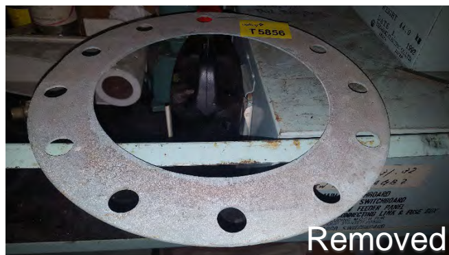
Photo 80 T5856 2nd Deck Storage Area 2nd Shelf from Fore - Gasket Loose (Blue) 'No Branding'
