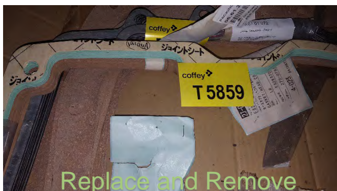
Photo 81 T5859 2nd Deck Storage Area, Above BD5 Cabinet – Gasket Loose 'Valqua' Black Font, Beige Background 350.01.01.072 (UMF)
