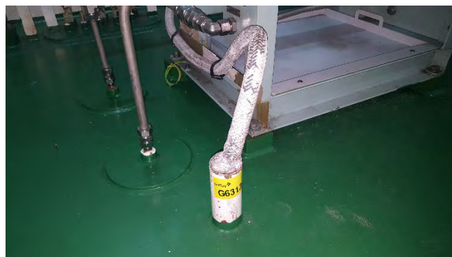
Photo 94 G6313 2nd Deck Nitrogen Space, No. B9 Solenoid Valve Box Deck Conduit – Bulkhead penetration insulation (Chrysotile)
