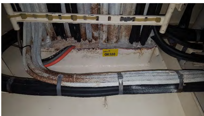
Photo 131 G6320 E Deck Electrical Cable Trunk Room, Cables Through Bulkhead - Bulkhead penetration insulation (Chrysotile)
