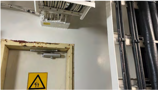
Photo 203 ZA9324 Void spaces in deck head, C deck fwd cross alley way (Chrysotile)
