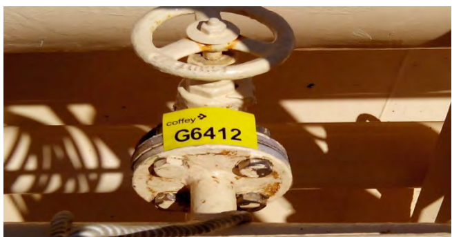
Photo 137 G6412 F Deck Flying Passage, Dome No.2, Air Supply Isolation Valve, Adjacent Fire Hydrant No.46 – Gasket (UMF)
