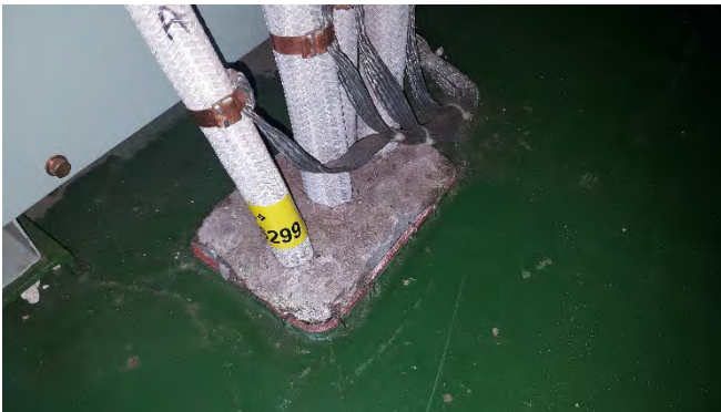
Photo 69 T5751 No. 1 Switch Board Room, Deck Conduit, Engine Service Transformer - Bulkhead penetration insulation (Chrysotile)
