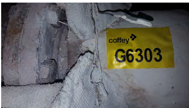
Photo 89 G6254 2nd Deck Steam Isolation Valve to Cargo Machinery Room – Lagging (Chrysotile)
