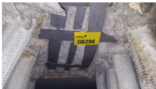
Photo 88 G6298 2nd Deck - No. 2 Switch Board Room, Deckhead Conduit – Bulkhead penetration insulation (Chrysotile)
