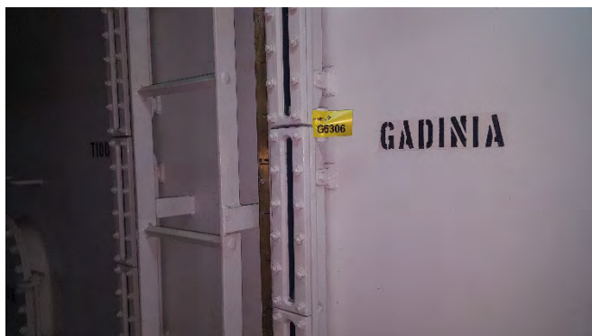
Photo 91 G6306 2nd Deck - Diesel Generator Lube Oil Tank Sight Level Glass, Horizontal Bracket – Gasket (UMF)
