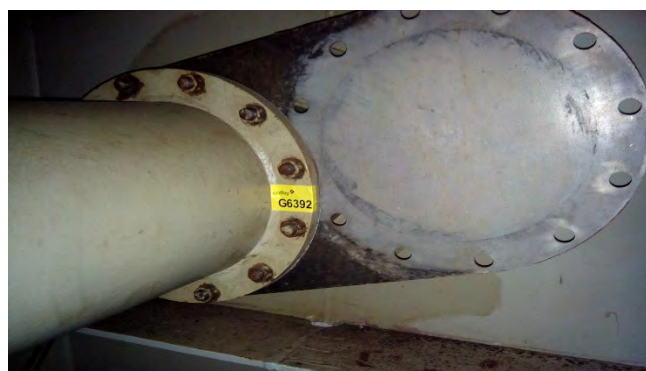
Photo 120 G6392 Upper Deck - Pipe Passage Port, Spectacle Piece Inlet Gas Flange, Frame 65 – Gasket (Chrysotile)
