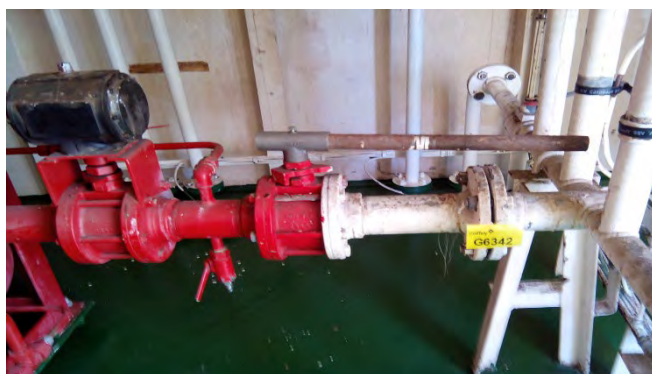
Photo 102 G6342 Upper Deck - Dry Chemical Unit Room, Aft, Outlet Flange From Storage - Gasket (Chrysotile)
