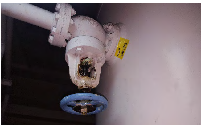
Photo 11 G6170 4 th Deck Engine Room, FWD Port, General Service Air Receiver Inlet Valve, Flange – Gasket (UMF)
