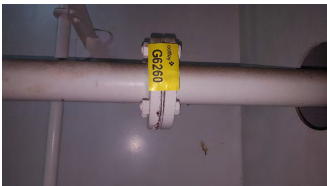
Photo 61 G6260 3rd Deck - Steering Gear, Fire Hydrant Line (FWD) Flange – Gasket (UMF)
