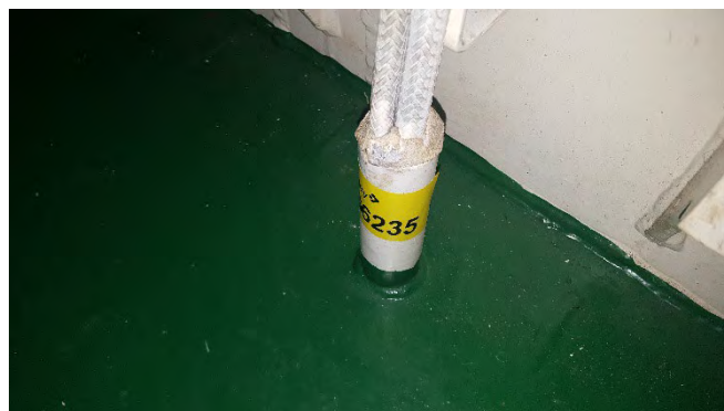
Photo 56 G6235 3rd Deck Lift Motor Room, Sealant to Conduit at Deck Level – Putty (Chrysotile)
