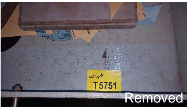
Photo 39 T5751 3rd Deck Workshop, Bulkhead penetration insulation Draws, First Draw (Labelled Off-Cuts)– Gasket (Chrysotile)
