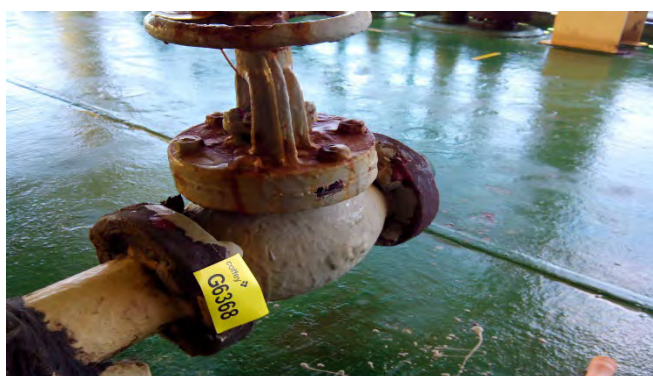
Photo 107 G6368 Upper Deck External, Starboard, Manifold Fresh Water From Shore Connection Inboard Valve Flange – Gasket (UMF)
