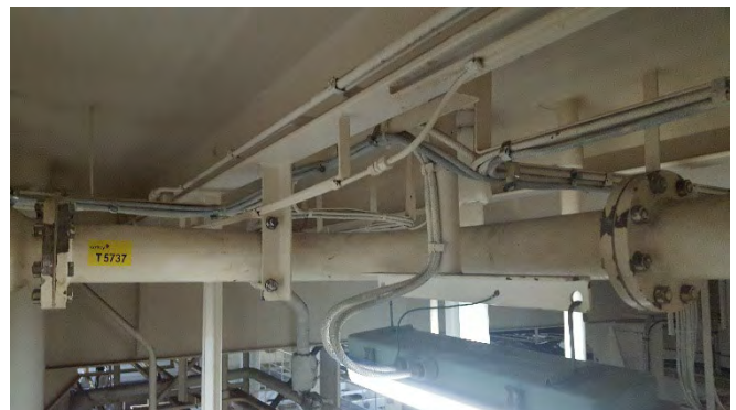
Photo 34 Refer to T5737 3rd Deck Workshop Mezzanine, Starboard, Diesel Oil Inlet Pipework to Fore– Gasket (White) (Chrysotile)
