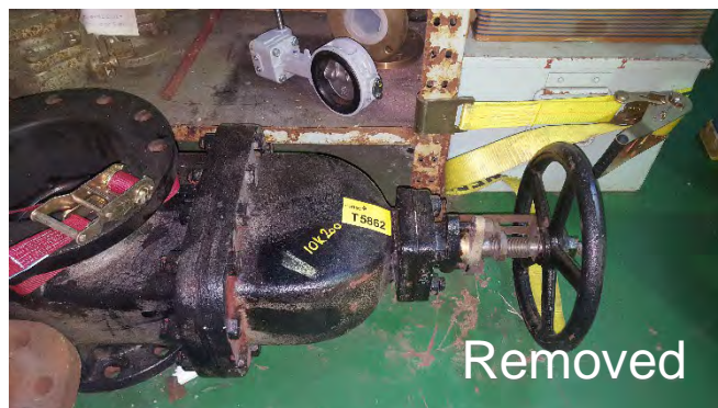
Photo 84 T5862 2nd Deck - Storage Area, Structural Column Adjacent 2nd Shelf from Fore – Gasket to Bonnet of Redundant Valve (Painted Black) (Chrysotile)
