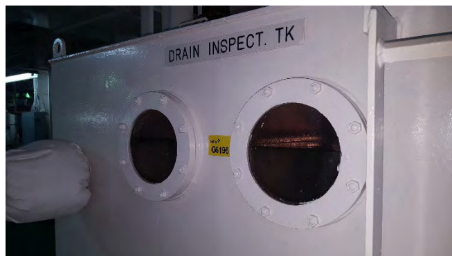
Photo 14 G6196 4 th Deck Engine Room, Starboard, FWD, Drain Inspection Tank, Inspection Glass Port – Gasket (UMF)
