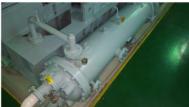
Photo 55 G6228 3rd Deck - Turbo Alternator, Cooling Water Outlet – Gasket Material (Chrysotile)
