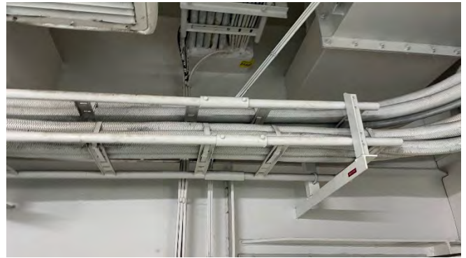
Photo 204 ZA9322 Bulkhead cable penetration putty material, Upper deck electrical cable trunk room (Chrysotile)
