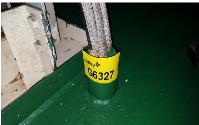
Photo 97 G6327 Upper Deck - Hydraulic Pump Unit Room (Ballast) Hydraulic Tank, Conduit Through Deck – Bulkhead penetration insulation (Presumed Positive) (Chrysotile)
