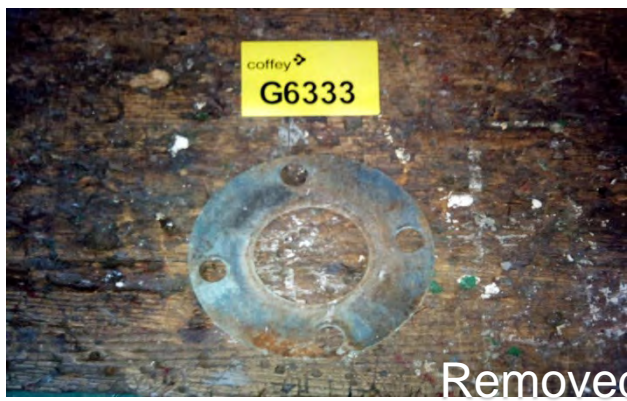
Photo 98 G6333 Upper Deck - External, Deck Workshop - Gasket Loose 'No Brand' (Blue) (UMF)
