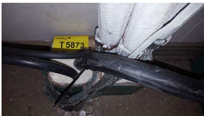
Photo 135 T5873 F Deck No.2 Equipment Room, Bulkhead penetration insulation (Off-White, Soft) (Presumed Positive) (Chrysotile)
