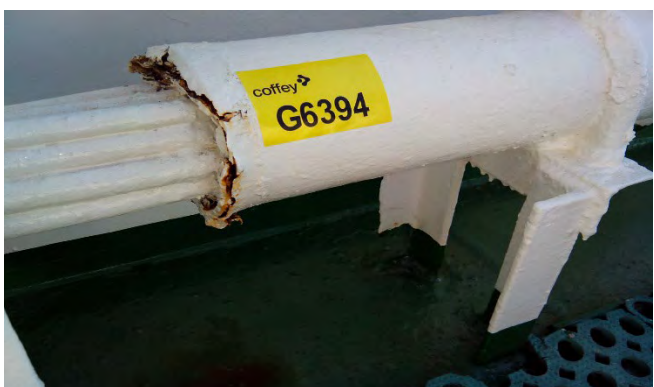
Photo 141 G6394 Nav. Bridge Starboard Bridge Wing – Bulkhead penetration insulation (Presumed Positive) (Chrysotile)
