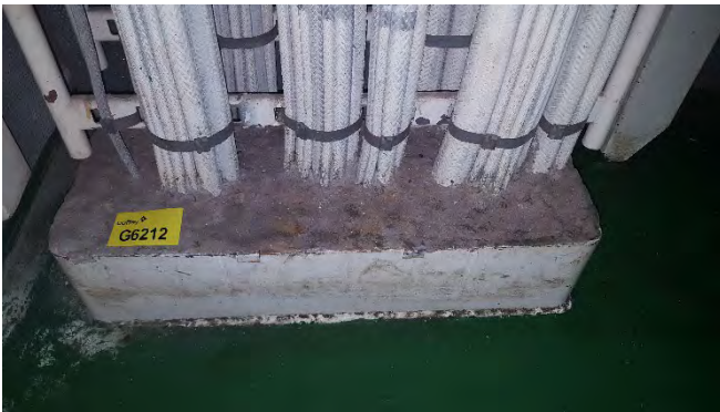
Photo 47 G6212 3rd Deck No.1 Diesel Alternator Room, Left of Inboard Door, Penetration – Bulkhead penetration insulation (Chrysotile)
