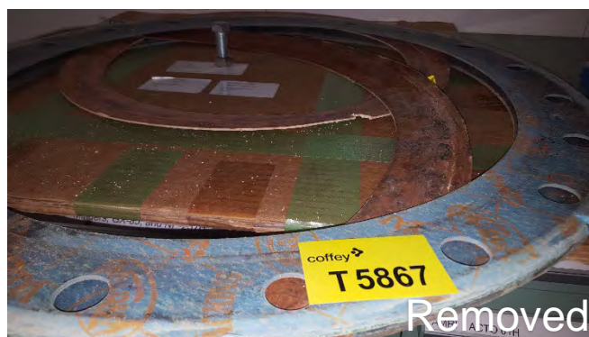
Photo 132 T5867 F Deck - No.2 Equipment Room, Aft Wall - Gasket Loose 'Valqua' (UMF)
