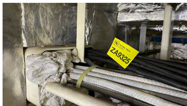
Photo 202 ZA9325 Bulkhead cable penetration putty material G deck electrical cable trunk room – Aft (Chrysotile)
