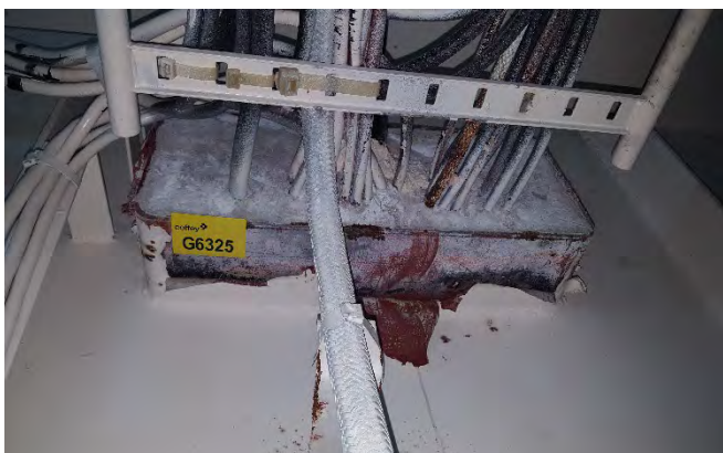
Photo 127 G6325 A Deck - Electrical Cable Room, Conduit Through Bulkhead – Bulkhead penetration insulation (Chrysotile)
