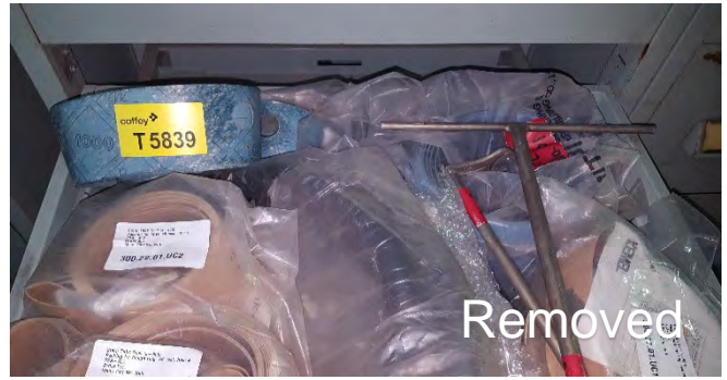
Photo 74 T5839 Storage Area, Drawer AL2, Stern Tube Seals - Gasket Loose t (Pink, Black Font, Tombo 1100) (Chrysotile)
