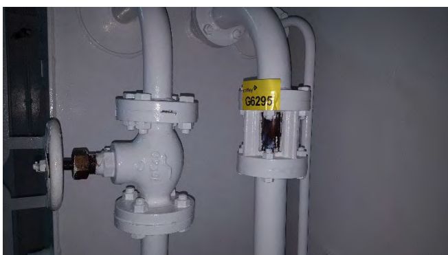
Photo 125 G6295 A Deck Incinerator Room, Diesel Oil Tank, Overflow Sight Glass Top Flange - Gasket (UMF)
