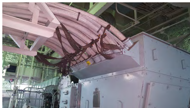
Photo 50 G6217 3rd Deck No.2 Diesel Alternator Room , Alternator Cabling Starboard Conduit – Putty (Chrysotile)
