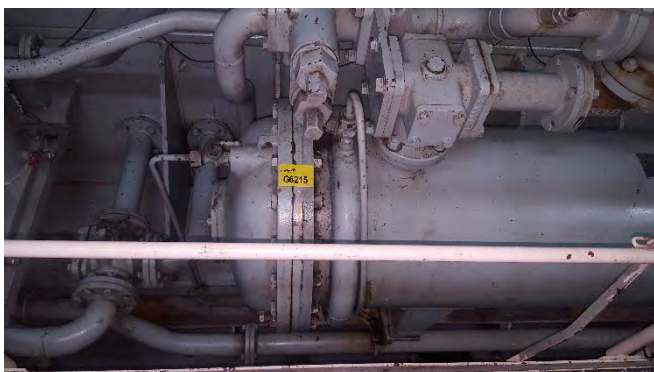
Photo 49 G6215 3rd Deck - No.1 Diesel Alternator Room , Lube Oil Cover, End Cover FWD – Gasket (UMF)
