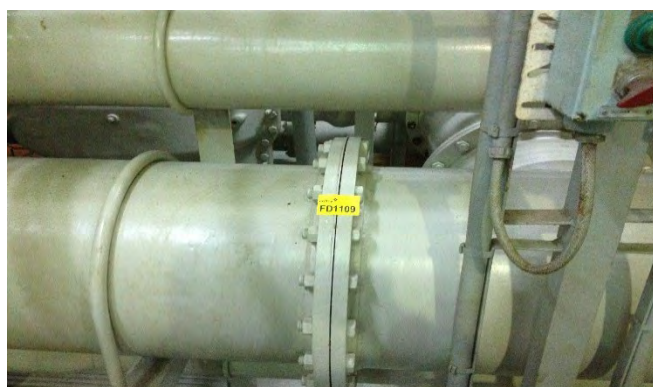
Photo 148 FD1109 Lower Deck, Seawater Cooling System Pipework Valves - Gasket (UMF)
