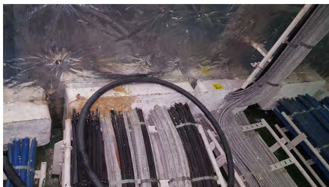
Photo 140 G6319 F Deck Electrical Cable Space, Starboard, Cables Through Bulk Head - Bulkhead penetration insulation (Chrysotile)
