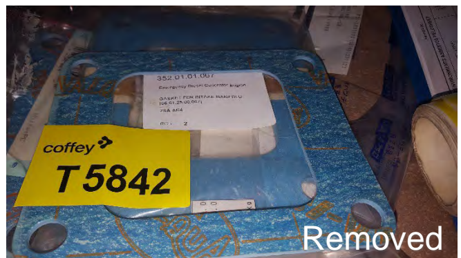
Photo 76 T5842 2nd Deck - Storage Area, Drawer, AE4 Emergency Generator - Gasket Loose 'Valqua' (Orange Font, Blue Backing) Japanese Symbols (UMF)
