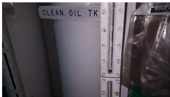
Photo 66 Refer to G6290 3rd Deck - Engine Room, Clean Oil Tank, Lube Oil Gravity Tank Level Sight Glass Flange - Gasket (Chrysotile)
