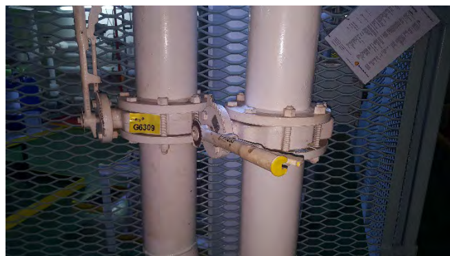
Photo 92 G6309 2nd Deck - Chemical Locker (Rear of), 2PA Valve (V0PJ234 Flange - Gasket (UMF)
