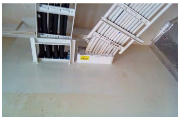
Photo 100 G6339 Upper Deck - Helicopter Rescue Equipment Store Penetration, – Bulkhead penetration insulation (Chrysotile)
