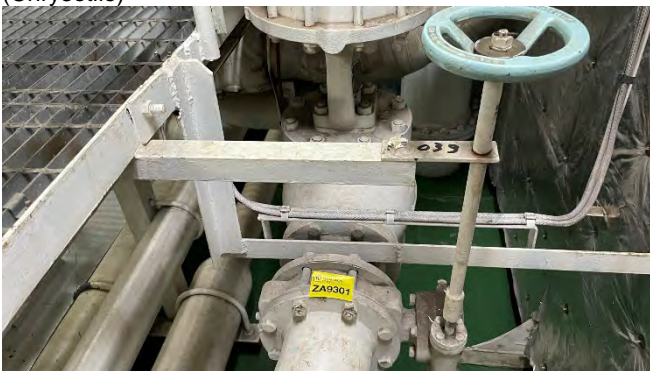
Photo 205 ZA9301 E/R DG Room 1, Cooling system inlet (Chrysotile)
