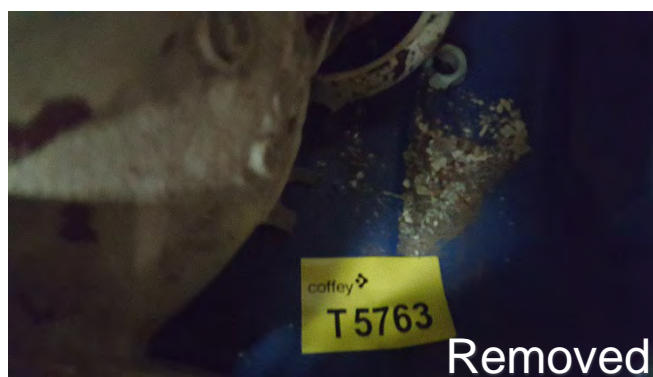
Photo 28 T5763 3rd Deck - Workshop Mezzanine, (In Blue Plastic Tub) – Gasket Fragments, Debris and Dust (Chrysotile)
