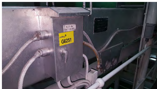
Photo 58 G6251 3rd Deck - Engine Room, Starboard No.2 Boiler, No.1 Retractable Soot Blower Power Box Conduit Sealant – Putty (Chrysotile)
