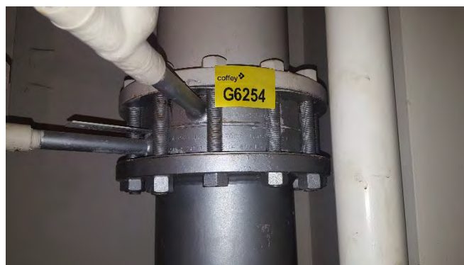
Photo 90 G6305 2nd Deck - Lube Oil Storage Tank Level Sight Glass, Top Bracket – (UMF)
