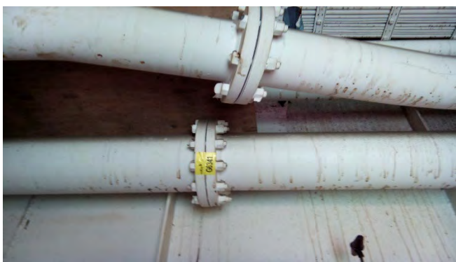
Photo 101 G6341 Upper Deck Chippy Store, Port, Overhead Pipework – Gasket (UMF)
