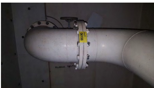
Photo 15 G6199 4 th Deck Engine Room, Fourth Deck, Aft, – Gasket (UMF)
