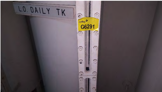
Photo 67 G6291 3rd Deck - Engine Room, Gardina 30 Oil Tank Sight Glass – Gasket (UMF)
