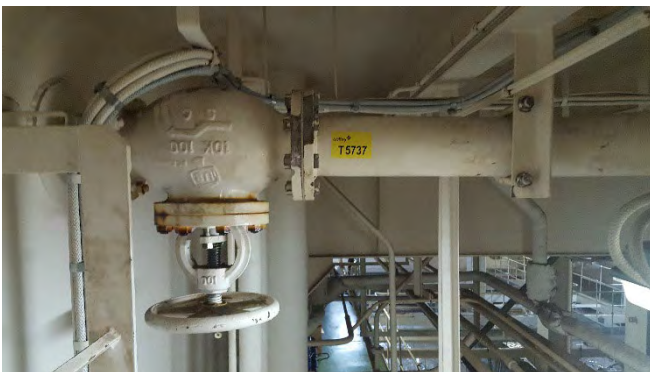
Photo 33 T5737 3rd Deck Workshop Mezzanine, Starboard, Fore, Diesel Oil Inlet (3 Way Valve) – Gasket (White) (Chrysotile)
