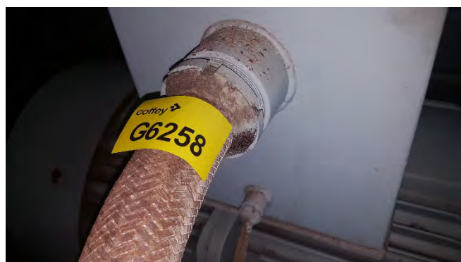
Photo 60 G6258 3rd Deck - Steering Gear, No.1 Hydraulic Motor Conduit Sealant - Putty (Chrysotile)
