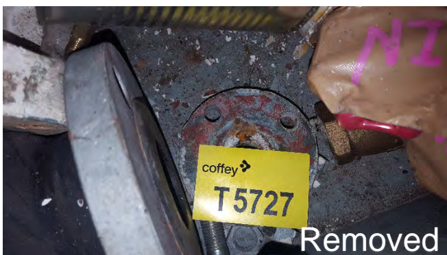
Photo 29 T5727 3rd Deck Workshop Mezzanine, Starboard, Fore, Adjacent Handrail, Stored Items, Throughout, to Small Flanges (Blue Metal Box) – Gasket Material (Blue, White Flecks, No Brand) Adhered to Valve (UMF)
