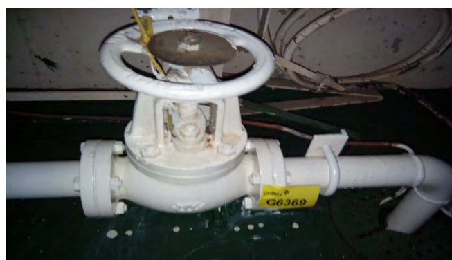
Photo 108 G6369 Upper Deck - Forecastle/Bosun Store, Port Bilge Suction Flange- Gasket (UMF)
