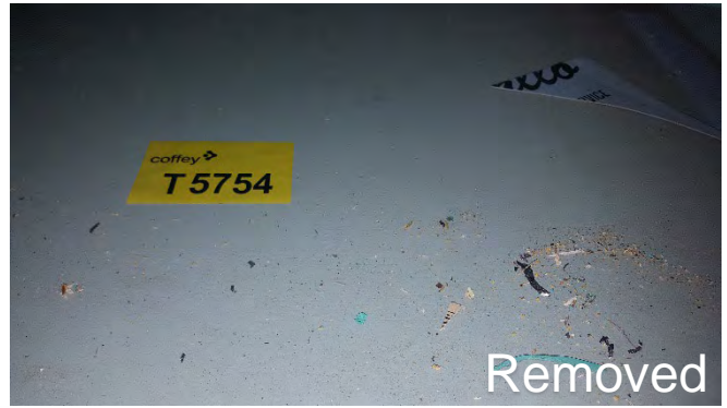
Photo 38 T5754 3rd Deck Workshop, Bulkhead penetration insulation Draws, Third Draw (Labelled 1.0 - 1.5mm) – Gasket Fragments, Debris and Dust (Chrysotile)
