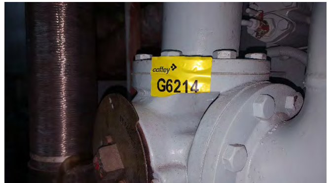
Photo 48 G6214 3rd Deck - No.1 Diesel Alternator Room, Charge Air Cooler Bypass Valve – Gasket (UMF)
