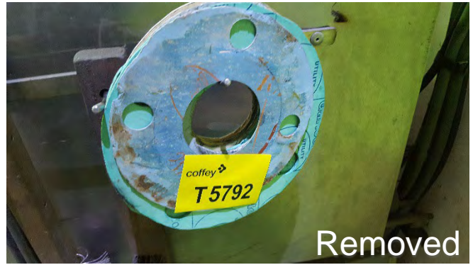
Photo 44 T5792 3rd Deck Workshop, Welders Bench – Loose Gasket 'Valqua' (Orange Font, Blue Backing) (UMF)
