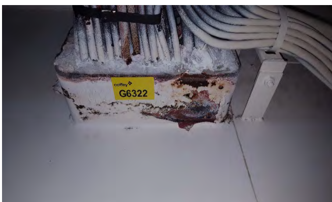
Photo 129 G6322 B Deck - Electrical Cable Trunk Room, Cables through Bulkhead – Bulkhead penetration insulation (Chrysotile)
