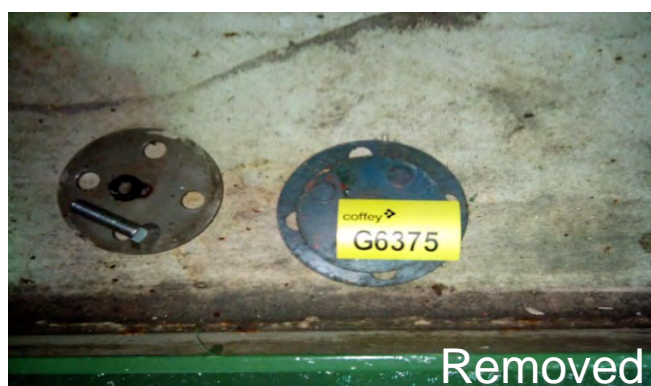
Photo 112 G6375 Upper Deck Forecastle/Bosun Store, to Storage Oil Tank Save - Gaskets Loose (UMF)
