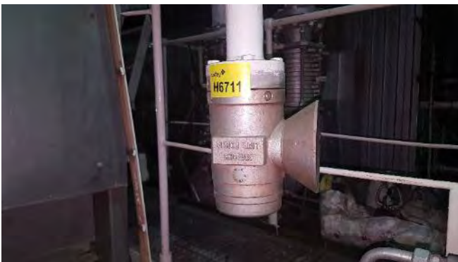
Photo 59 H6711 3rd Deck, Burner Tops, Starboard Boiler Periscope, Gasket (Chrysotile)
