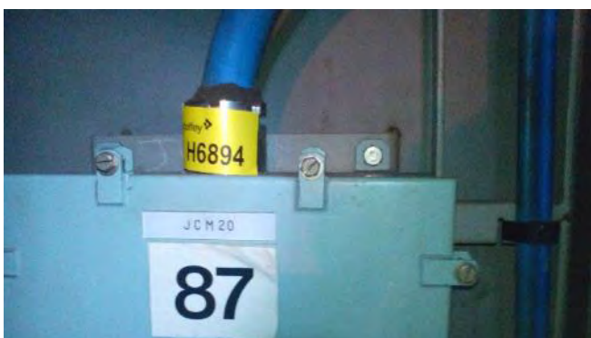
Photo 125 G6894 Upper Deck, Port Passage, Electrical Cabinet JCM-20 Frame 87, Putty (Chrysotile)
