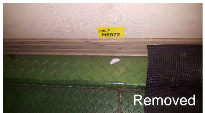
Photo 144 H6972 F Deck, No.1 Equipment Room, Port FWD, Debris (Chrysotile)
