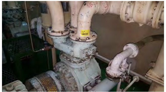
Photo 110 G6838 Upper Deck, Fo'c'sle/Bosons Store, Hydraulic Pump No.2 Suction Flange, Gasket (Chrysotile)
