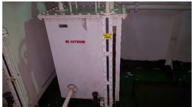
Photo 52 G6688 3rd Deck, Steering Flat, Overflow Tank Level Gauge Glass, Gasket (Chrysotile)
