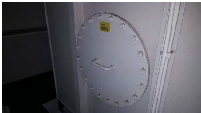
Photo 80 H6759 2nd Deck, Gen. Eng. L.O. Renovating Tank Side Manhole, Gasket (Chrysotile)
