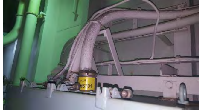
Photo 56 G6701 3rd Deck, Steering Flat, Power Cable Conduit Aft Winch Electrical Cabinet, Putty (Chrysotile)
