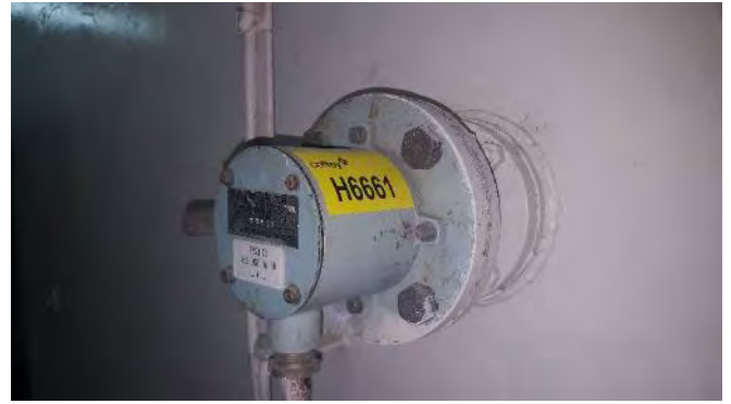
Photo 32 H6661 3rd Deck, Engine Room, No.1 Distilled Water Tank Low Level Switch Flange, Gasket (Chrysotile)
