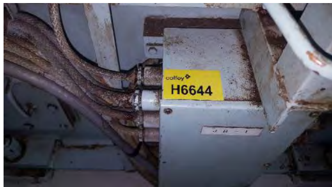
Photo 26 H6644 3rd Deck, Engine Room, Diesel Alternator Junction Box JB-1, Putty (Chrysotile)
