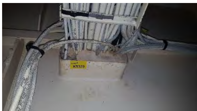
Photo 186 K5329 3rd Deck, Workshop Mezzanine, Port Aft Penetration, Packing (Grey/Cream) (Chrysotile)
