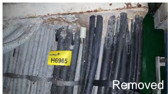
Photo 138 H6965 F Deck, Electric Cable Space, Starboard Bulkhead (Around Cables), Debris & Dust (Grey) (Chrysotile)
