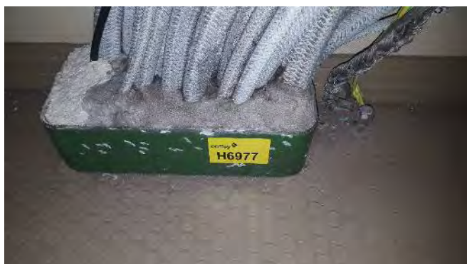
Photo 149 H6977 F Deck, No.2 Equipment Room, Penetration Through Deck, Packing (Grey) (Chrysotile)
