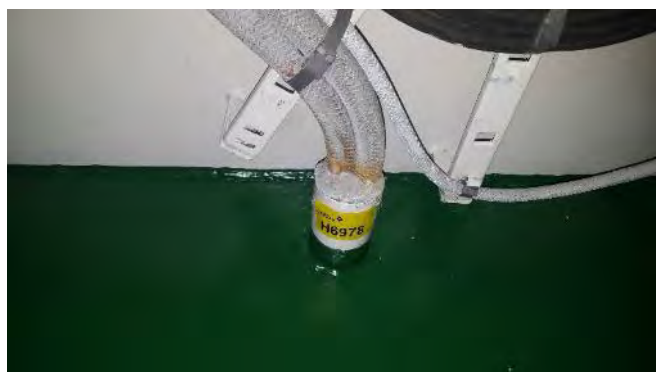
Photo 150 H6978 E Deck, Electrical Cable Trunk Room, Inboard Deck Penetration, Packing (Grey) (Chrysotile)
