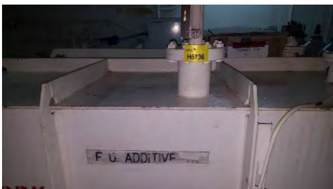
Photo 69 H6736 2nd Deck, Port, Fuel Oil Additive Tank Sight Level Gauge, Gasket (Chrysotile)
