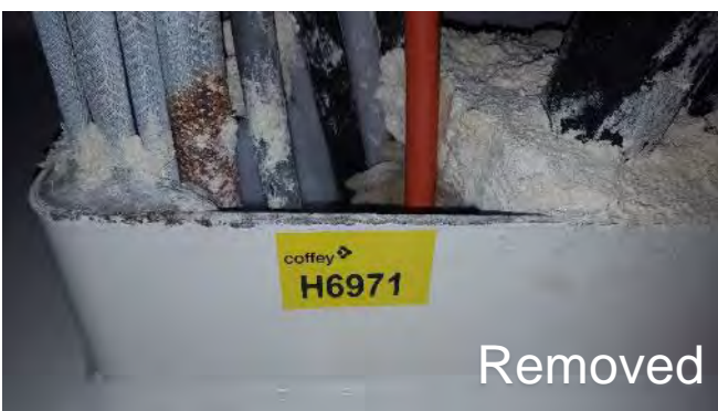
Photo 143 H6971 F Deck, Electrical Cable Trunking, Inboard Deck Head, Debris (Chrysotile)
