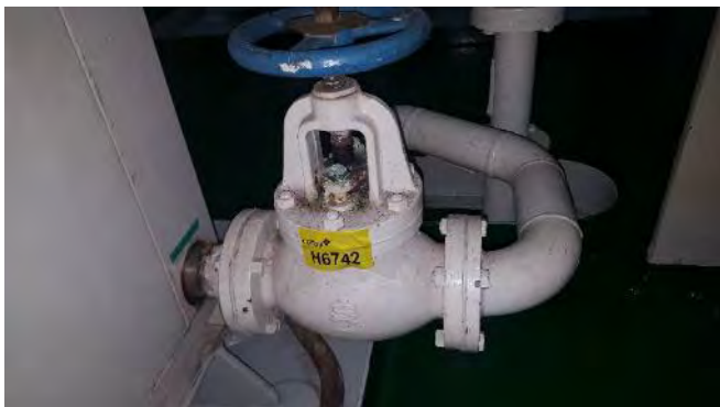
Photo 71 H6742 2nd Deck, Port, Package Cooler Inlet Valve Flange, Gasket (Chrysotile)
