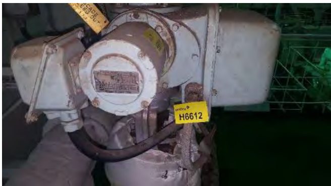
Photo 19 H6612 4th Deck, Engine Room, No.2 Cascade Controller Conduit, Putty (Chrysotile)
