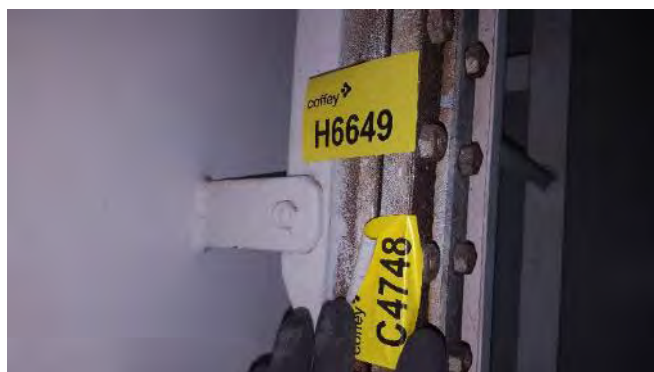
Photo 28 H6649 3rd Deck, Engine Room, Turbine Oil Gravity Tank Level Sight Glass, Gasket (Chrysotile)
