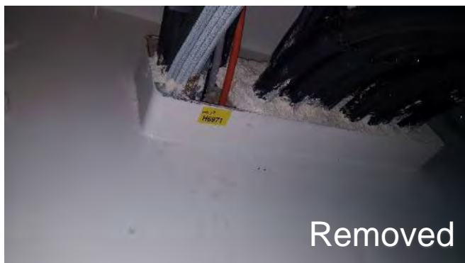
Photo 145 H6973 F Deck, No.1 Equipment Room, Starboard Aft, Debris & Dust (Chrysotile)
