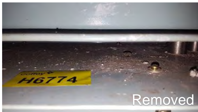
Photo 86 H6774 2nd Deck, No.2 Main Switchboard Room (O/B) on Top of Electrical Cabinet, Mixed Debris (Chrysotile)
