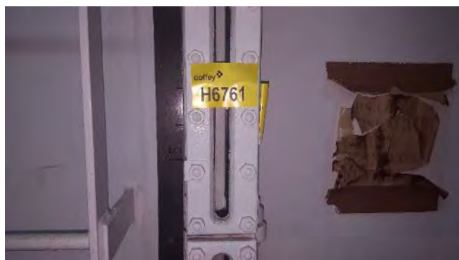
Photo 82 H6761 2nd Deck, Gen. Eng. L.O. Purifying Tank Level Gauge Glass, Gasket (Chrysotile)
