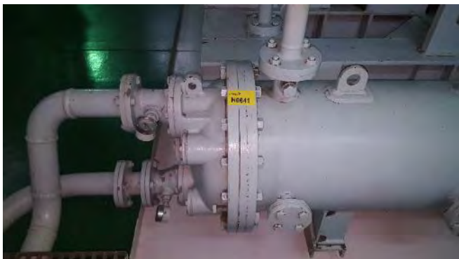
Photo 25 H6641 3rd Deck, Engine Room, Diesel Alternator L.O. Cooler End Cover, Gasket (Chrysotile)
