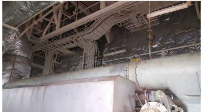
Photo 50 H6685 3rd Deck, No.2 Diesel Generator Room, Exhaust Gasket at Charge Air Cooler, Gasket (Chrysotile)
