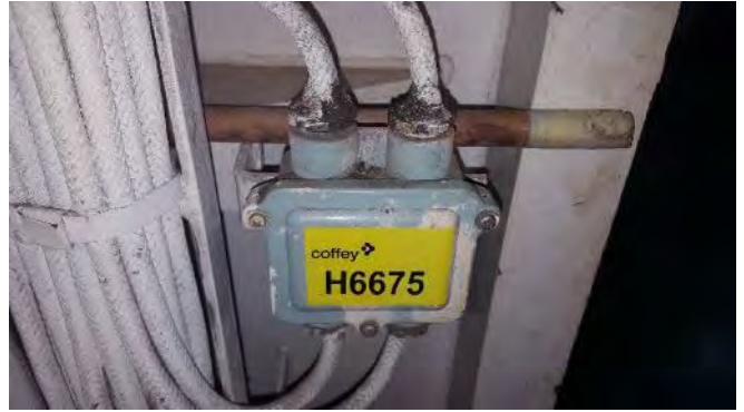
Photo 38 H6675 3rd Deck, IGG Room, Junction Box Adj. Door, Putty (Chrysotile)
