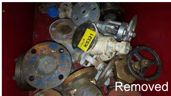
Photo 182 K5321 2nd Deck, Workshop Loft, Large Yellow Metal Box White Valve, Gasket Adhered to Valve (Chrysotile)
