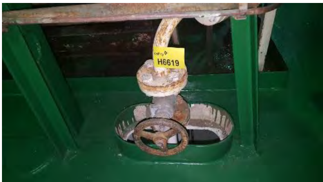
Photo 21 H6619 4th Deck, Engine Room, Electric Lighting EL7 Conduit, Putty (Chrysotile)
