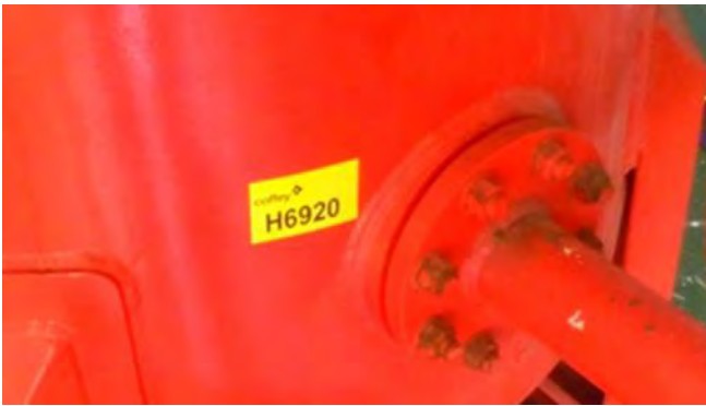
Photo 133 H6920 Upper Deck, No.3 Dry Chemical Powder Room Vessel Pipework Outlet Flange to Manifold, Gasket
