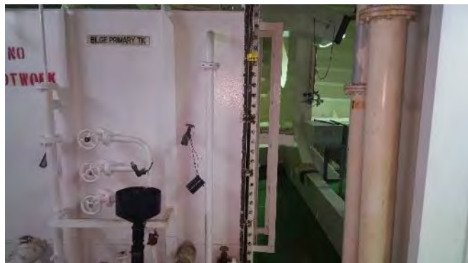
Photo 20 H6617 4th Deck, Engine Room, Bilge Primary Tank Level Indicator, Sight Glass, Gasket (Chrysotile)
