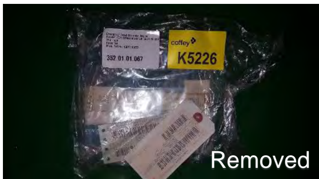
Photo 155 K5226 2nd Deck, 2SA, AE4 352.02.02.067 Emergency Diesel Generator, Gasket (Valqua Blue Backing with Orange Font) for intake Manifold Daihatsu 0661 12500 067 (UMF)
