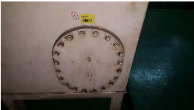
Photo 113 G6841 Upper Deck, Fo'c'sle/Bosons Store, Hydraulic Pump No.4 Suction Flange, Gasket (Chrysotile)
