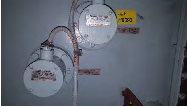
Photo 55 G6693 3rd Deck, Steering Flat, Starboard Header Tank Level Switch, Gasket (Chrysotile)
