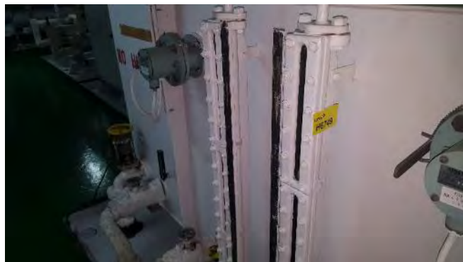
Photo 72 H6749 2nd Deck, Starboard, Aux. L.O. Purifying Tank (Small) & Aux L.O. Renovation Tank Sight Level Gauge, Gasket (Chrysotile)
