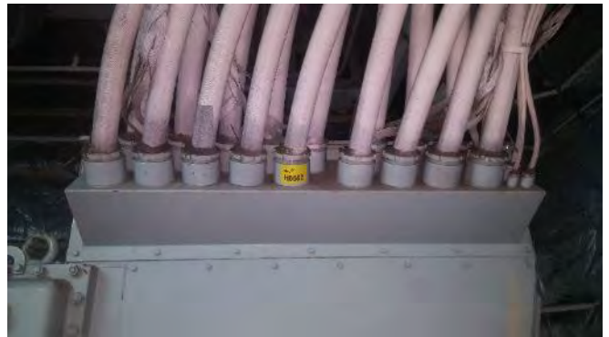
Photo 42 H6682 3rd Deck, No.2 Diesel Generator Room, Power Cables from Alternator, Putty (Chrysotile)
