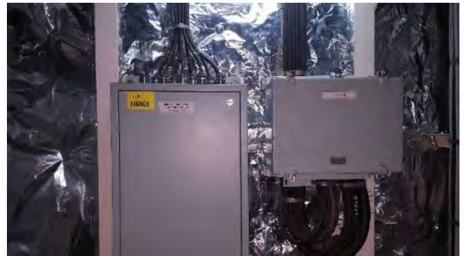
Photo 142 H6969 F Deck, Electrical Cable Trunking, Lighting Power Board "LO3", Putty (Chrysotile)
