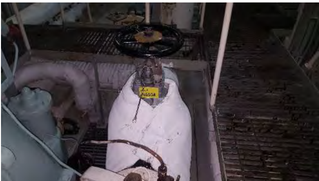
Photo 17 H6604 4th Deck, Purifier Room, HFO Transfer Pump Cross Connection Valve Bonnet, Gasket (Chrysotile)
