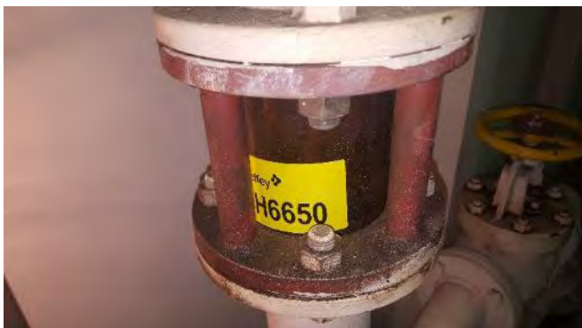
Photo 29 H6650 3rd Deck, Engine Room, Turbine Oil Gravity Tank Level Overflow Sight Glass, Gasket (Chrysotile)
