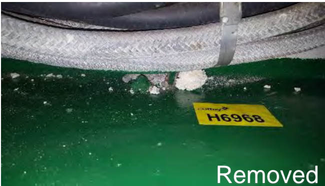
Photo 141 H6968 F Deck, Electric Cable Space, Below Inboard Deck Head, Debris & Dust (Chrysotile)
