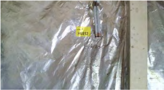
Photo 129 H6912 Upper Deck, Deck Rope Store (Starboard Aft), Packing (Chrysotile)
