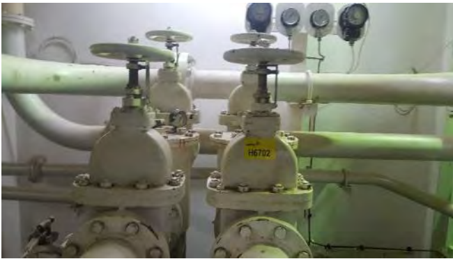
Photo 57 H6702 3rd Deck, Steering Flat, Hydraulic Valve Bonnet, Gasket (Chrysotile)
