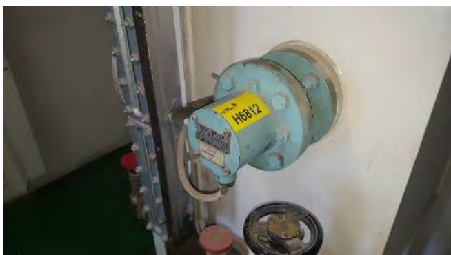
Photo 99 G6812 A Deck, Incinerator Room, Diesel Tank – Low Level Switch, Gasket (Chrysotile)
