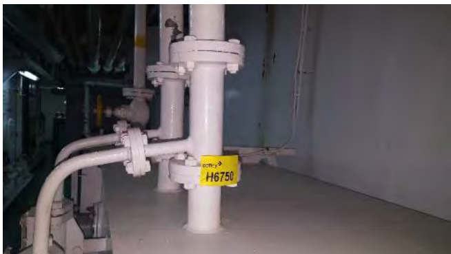
Photo 73 H6750 2nd Deck, Starboard, L.O. Renovation Tank (Small) Filling Line, Gasket (Chrysotile)
