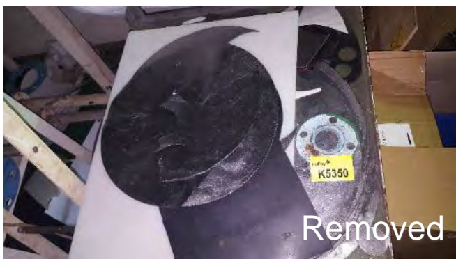
Photo 191 K5350 3rd Deck, Workshop, Graphite Stand, Gasket Loose "Tombo" (Blue Backing White Specks Black Font) (Chrysotile)
