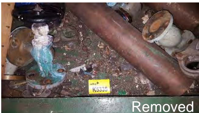
Photo 187 K5335 3rd Deck, Workshop, Work Bench Adjacent Wooden Block, Caged Floor Area (Aft), Debris (Mixed) (Chrysotile)
