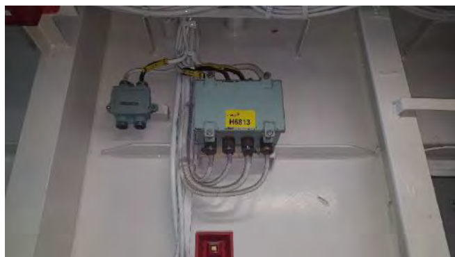
Photo 100 G6813 A Deck, Incinerator Room, Junction Box, FWD Bulkhead Adj. 1IF 154C Box, Putty (Chrysotile)
