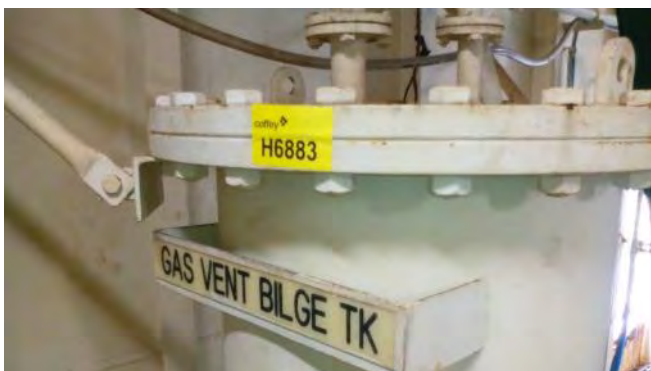
Photo 121 G6883 Upper Deck, Cargo Motor Room, Gas Vent Bilge Tank Cover, Gasket (Chrysotile)
