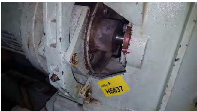
Photo 23 H6637 3rd Deck, Lift Motor Room, Braking System Friction Material, Lining (Chrysotile)
