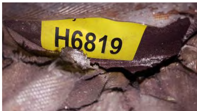
Photo 102 G6819 B Deck, Engine Room, Incinerator Exhaust Trunking (Adj. No.1 Fan Room Exhaust), Gasket (Chrysotile)
