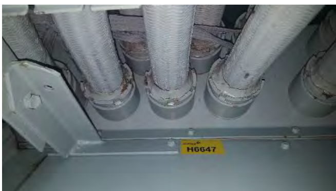
Photo 27 H6647 3rd Deck, Engine Room, Diesel Alternator Electrical (x16) Cables Outlet, Putty (Chrysotile)
