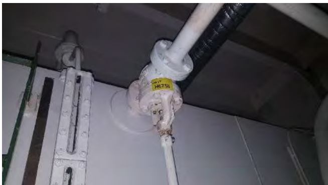
Photo 79 H6758 2nd Deck, D/G L.O. Storage Tank Filling Valve, Gasket (Chrysotile)
