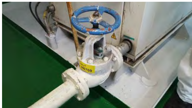
Photo 84 H6769 2nd Deck, Package Cooler Starboard Cooling Inlet Valve, Gasket (Chrysotile)
