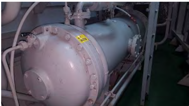
Photo 97 G6799 Upper Deck, Emergency Generator Room L.O. End Cover, Gasket (Chrysotile)
