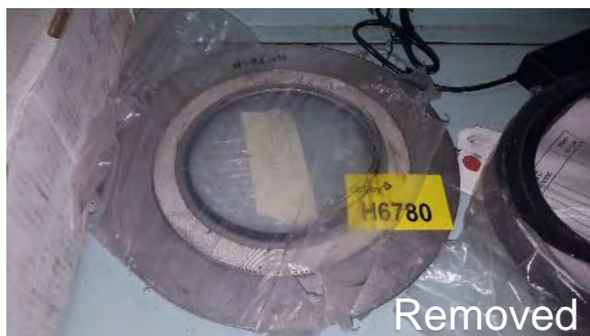
Photo 90 H6780 2nd Deck, Control Room, Above DB3 Dist. Panel AC100v, Large Spiral Bound Gasket (White Sealing Element) (Chrysotile)
