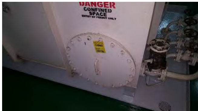
Photo 68 H6735 2nd Deck, Port, Fuel Oil Additive Tank Manhole Cover, Gasket (Chrysotile)
