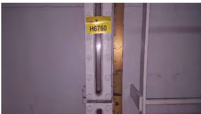
Photo 81 H6760 2nd Deck, Gen. Eng. L.O. Renovating Tank Level Gauge Glass, Gasket (Chrysotile)
