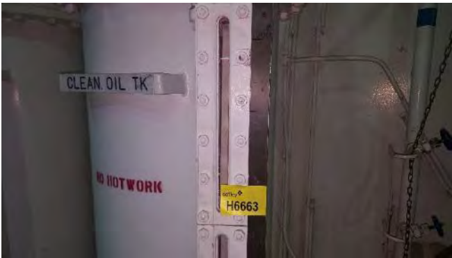
Photo 33 H6663 3rd Deck, Engine Room, Clean Oil Tank Level Sight Glass, Gasket (Chrysotile)
