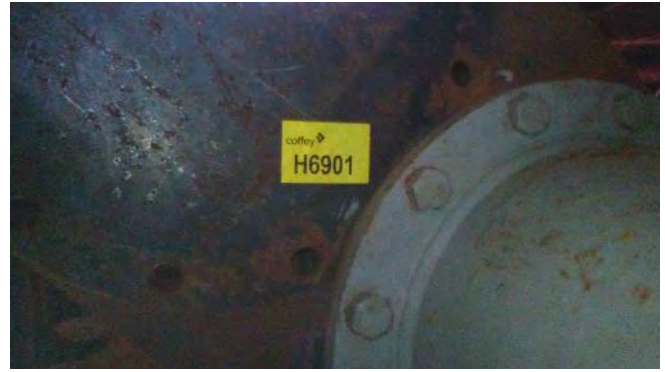
Photo 128 H6901 Upper Deck, Port Passage, Spectacle Piece Starboard Frame 66, Gasket (UMF)
