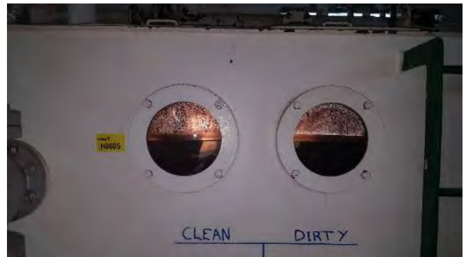
Photo 18 H6605 4th Deck, Engine Room, Hotwell/Observation Tank Viewing Glass Gasket (Chrysotile)
