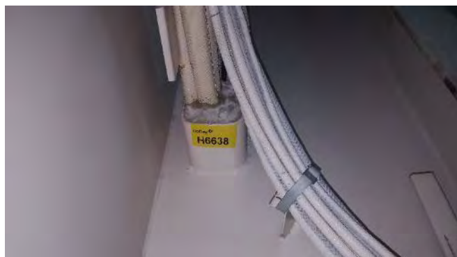
Photo 24 H6638 3rd Deck, Lift Motor Room, Penetration, Packing (Chrysotile)
