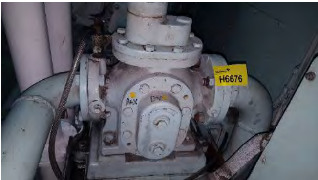
Photo 39 H6676 3rd Deck, No.1 Diesel Generator Room, L.O. Priming Pump Outlet Flange, Gasket (Chrysotile)
