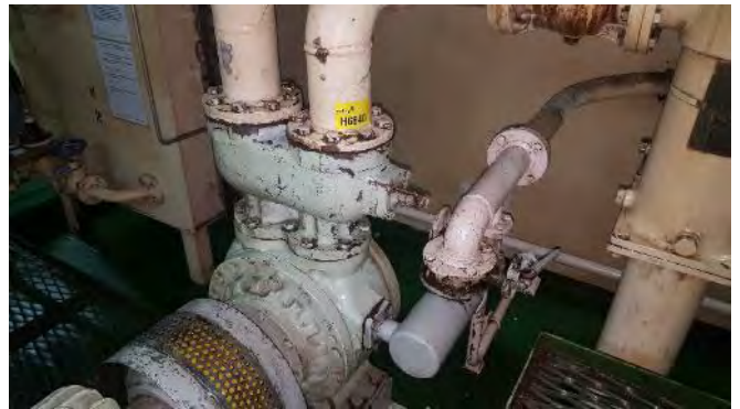
Photo 112 G6840 Upper Deck, Fo'c'sle/Bosons Store, Hydraulic Pump No.4 Suction Flange, Gasket (Chrysotile)
