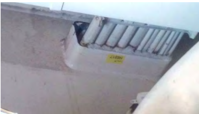
Photo 131 H6917 Upper Deck, Shipwright Store, Port Side Aft Through FWD Bulkhead, Packing (Chrysotile)
