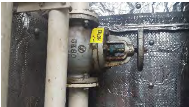
Photo 91 H6783 Upper Deck, Air Handling Room, Swimming Pool Drain Valve, Gasket (Chrysotile)
