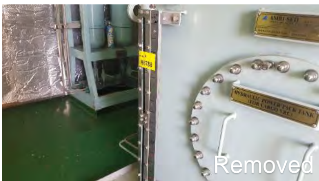
Photo 93 G6788 Upper Deck, Hydraulic Room, Cargo Power Pack Level Sight Glass, Gasket (Chrysotile)
