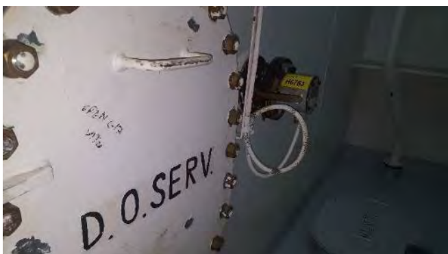
Photo 75 H6753 2nd Deck, Diesel Oil Service Tank Float Level Switch (x3), Gasket (Chrysotile)
