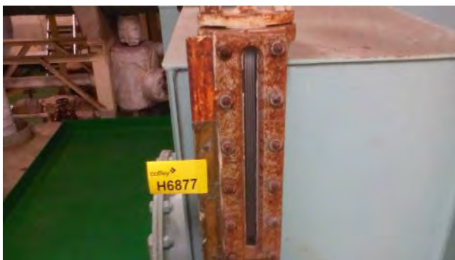
Photo 119 H6877 Upper Deck, Cargo Motor Room, L.O. Storage Tank Level Gauge Sight Glass, Gasket (Chrysotile)
