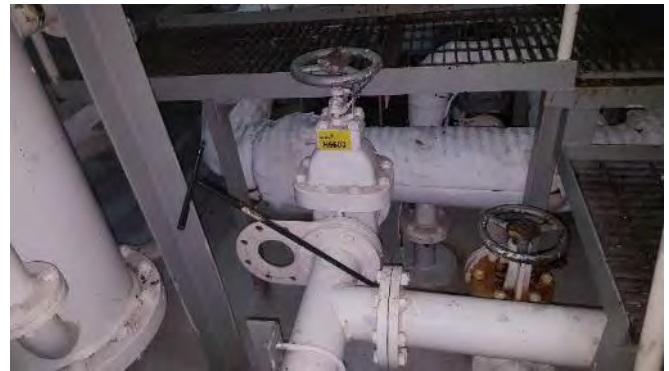
Photo 16 H6603 4th Deck, Purifier Room, D.O. Transfer Pump Cross Connection Valve Bonnet, Gasket (Chrysotile)
