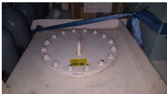
Photo 70 H6740 2nd Deck, Port, Fuel Oil Additive Tank Manhole Cover (Top), Gasket (Chrysotile)
