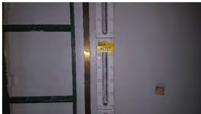
Photo 78 H6757 2nd Deck, D/G L.O. Storage Tank Level Gauge Glass, Gasket (Chrysotile)
