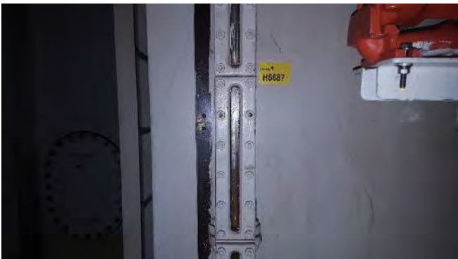
Photo 51 H6687 3rd Deck, Steering Flat, Transfer Oil Tank Level Gauge Glass, Gasket (Chrysotile)
