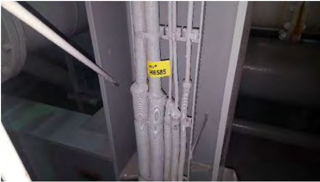
Photo 13 H6585 Tank Top/Lower Deck, Engine Room, Between No.1 & No.2 Main C.C.S Cooling S.W. Pumps, Putty (Chrysotile)
