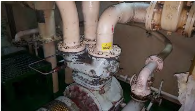
Photo 111 G6839 Upper Deck, Fo'c'sle/Bosons Store, Hydraulic Pump No.3 Suction Flange, Gasket (Chrysotile)
