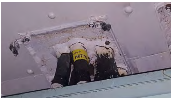
Photo 87 H6776 2nd Deck, No.1 Main Switchboard Room, Penetration to Deck Head, Packing (Chrysotile)
