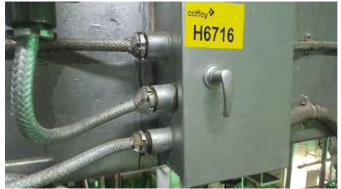
Photo 62 H6716 2nd Deck, Engine Room, Port Boiler No.1 Retractable Soot Blower Power Junction Box, Putty (Chrysotile)
