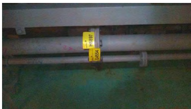
Photo 126 H6897 Upper Deck, Port Passage, Pipework Air Line Frame 66, Gasket (Chrysotile)
