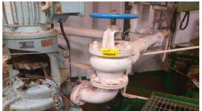
Photo 114 G6864 Upper Deck, Cargo Motor Room, No.1 Freshwater Pump Discharge Valve Casing, Gasket (Chrysotile)
