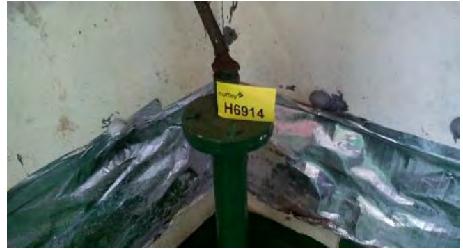
Photo 130 G6914 Upper Deck, B.A. Locker (Starboard Aft) Cable Conduit Pipe to Deck, Putty (Chrysotile)
