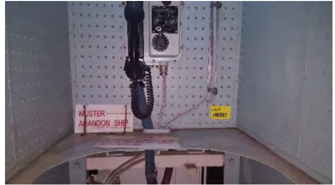
Photo 14 H6587 Tank Top/Lower Deck, Engine Room, Telephone Booth - Perforated Cladding, Fibre Board (Chrysotile)
