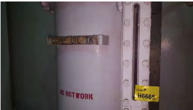
Photo 35 H6665 3rd Deck, Engine Room, Compressor Oil Tank Level Sight Glass, Gasket (Chrysotile)
