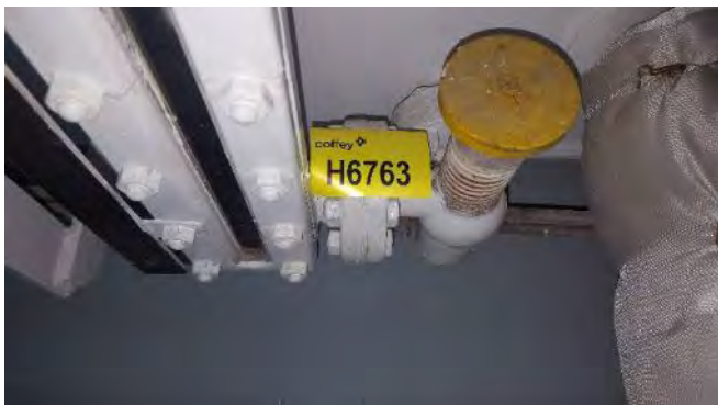
Photo 83 H6763 2nd Deck, Gen. Eng. L.O. Purifying Tank Level Gauge Glass Valve, Gasket (Chrysotile)
