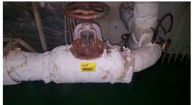
Photo 36 H6667 3rd Deck, IGG Room, HFO Tank Steam Heating Valve Flange, Gasket (Chrysotile)
