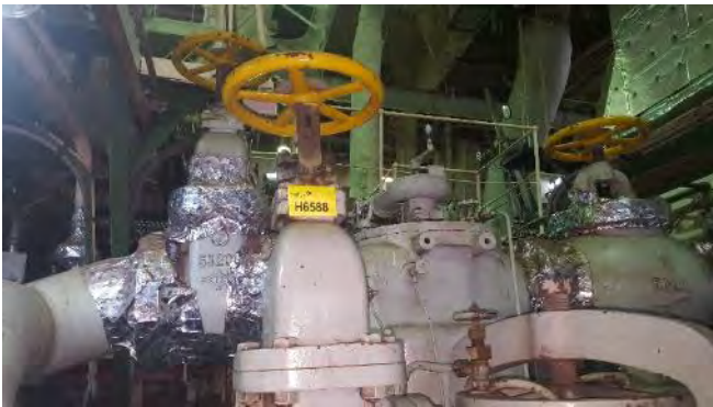
Photo 15 H6588 Tank Top/Lower Deck, Engine Room, Main L.O. Filter Bypass Valve, Gasket (Chrysotile)
