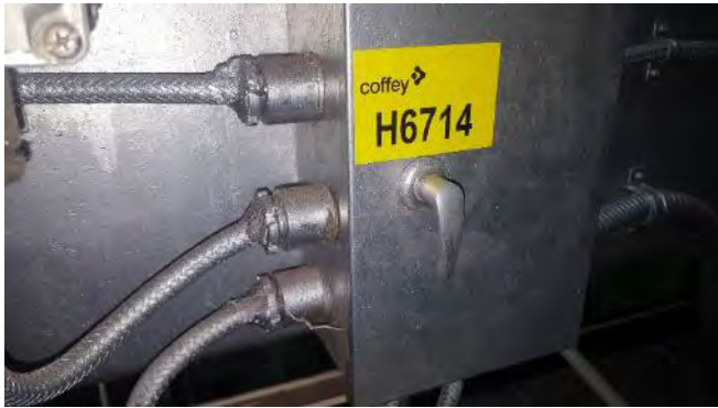
Photo 61 H6714 2nd Deck, Engine Room, Starboard Boiler No.1 Retractable Soot Blower Power Junction Box, Putty (Chrysotile)
