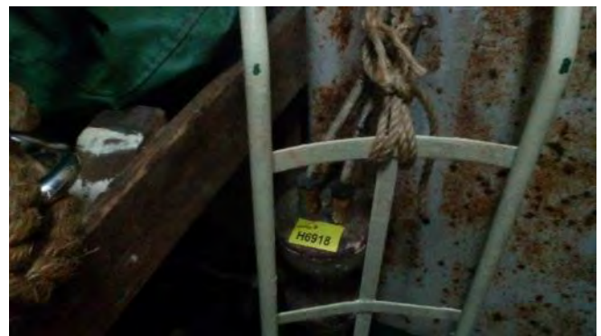
Photo 132 H6918 Upper Deck, Boat Gear Locker, Cable Penetration to Deck via Steel Conduit, Putty (Chrysotile)
