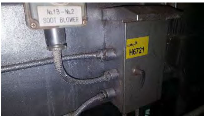
Photo 63 H6721 3rd Deck, Engine Room, Port Boiler No.1 Retractable Soot Blower Power Junction Box, Putty (Chrysotile)
