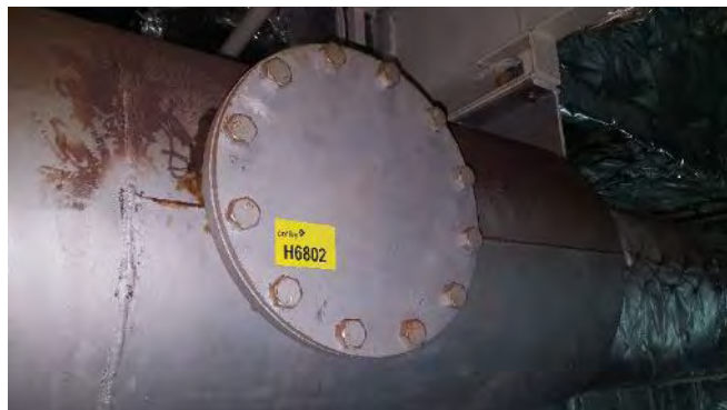
Photo 98 G6802 Upper Deck, Emergency Generator Room Exhaust Trunking Manhole, Gasket (Chrysotile)
