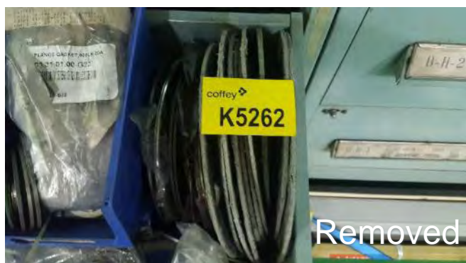
Photo 162 K5262 2nd Deck, 2SA, BJ2, Gaskets Loose (Various Grey Sizes) (Chrysotile)
