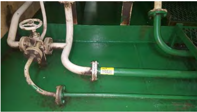
Photo 109 G6835 Upper Deck, Fo'c'sle/Bosons Store, Pipework to Transfer Oil Tank, Gasket (Chrysotile)
