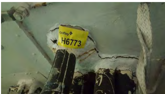
Photo 85 H6773 2nd Deck, No.2 Main Switchboard Room (O/B) Penetration to Deck Head, Putty (Chrysotile)
