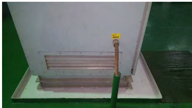
Photo 22 H6632 4th Deck, Engine Room, Hychlorinator Power, Inlet, Putty (Chrysotile)
