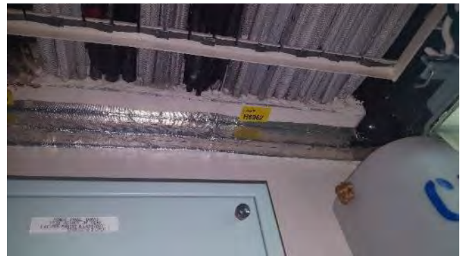
Photo 136 G6962 G Deck, Cable Trunk Room (CRYOS) FWD Bulkhead Penetration, Packing (Chrysotile)
