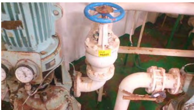
Photo 115 H6865 Upper Deck, Cargo Motor Room, No.2 Freshwater Pump Discharge Valve Casing, Gasket (Chrysotile)
