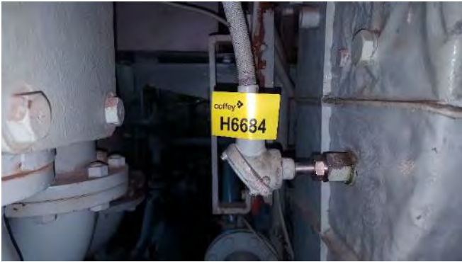
Photo 49 H6684 3rd Deck, No.2 Diesel Generator Room, Temperature Sensor - Charge Air Cooler, Gasket (Chrysotile)
