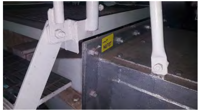
Photo 58 H6707 3rd Deck, Port Gas Hood, Boiler Gas Valve, Flange, Gasket (Chrysotile)
