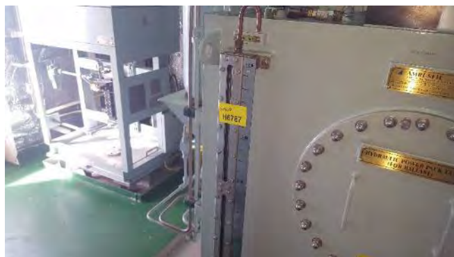
Photo 92 G6787 Upper Deck, Hydraulic Room, Ballast Power Pack Level Sight Glass, Gasket (Chrysotile)
