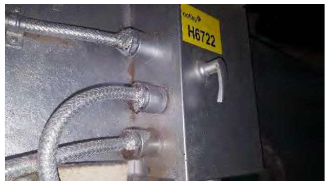
Photo 64 H6722 3rd Deck, Engine Room, Starboard Boiler No.1 Retractable Soot Blower Power Junction Box, Putty (Chrysotile)
