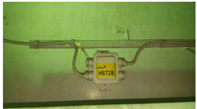
Photo 66 H6728 2nd Deck, Chemical Locker, Halogen Light Junction Box, Putty (Chrysotile)
