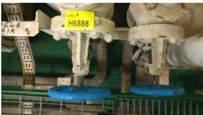
Photo 123 H6888 Upper Deck, Cargo Motor Room, Cooling Water Outlet From Drain Cooler, Gasket (Chrysotile)
