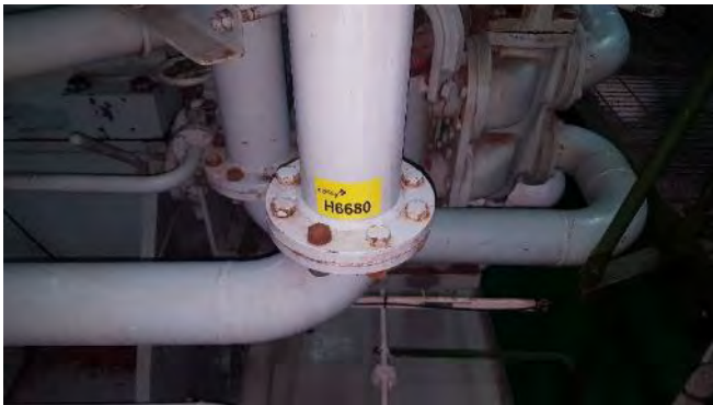
Photo 41 H6680 3rd Deck, No.1 Diesel Generator Room, Cooling Water Line - L.O. Cooler Inlet Flange, Gasket (Chrysotile)
