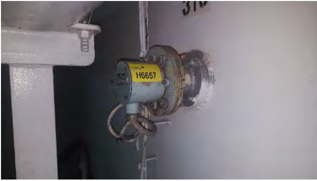
Photo 31 H6657 3rd Deck, Engine Room, Port Domestic F.W. Tank Low Level Switch Flange, Gasket (Chrysotile)
