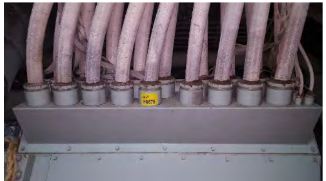
Photo 40 H6678 3rd Deck, No.1 Diesel Generator Room, Power Cables from Alternator, Putty (Chrysotile)
