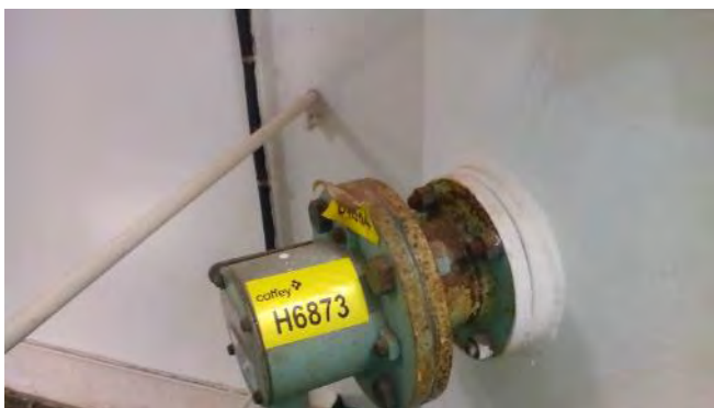
Photo 117 H6873 Upper Deck, Cargo Motor Room, AUX.CCS.F.W.EXP.TK Float Switch, Gasket (Chrysotile)
