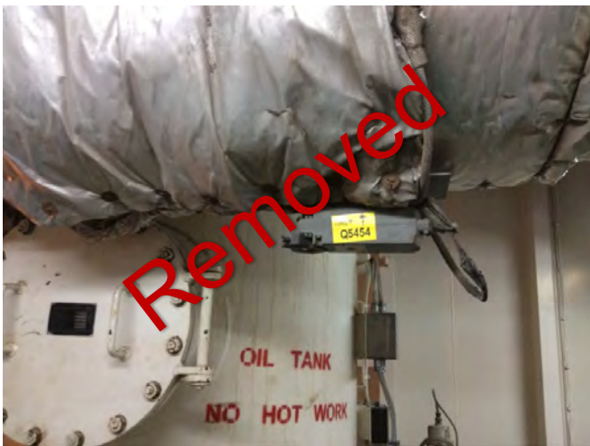
Photo 47 Q5454 A Deck – Incinerator Room – Incinerator Flue Incinerator Flue At Damper Inlet gasket
