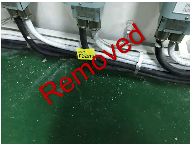
Photo 85 FD2510 F Deck – Electrical Cable Store – Aft, Deck Head Penetration Material Debris (Chrysotile)
