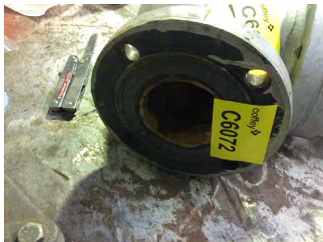
Photo 10 C6072 3rd deck - engine room workshop aft - welding bay Valve flange Valqua 1500 gasket
