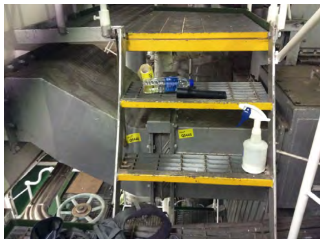
Photo 14 Q5445 2nd deck - engine room- starboard boiler gas hood expansion piece out
