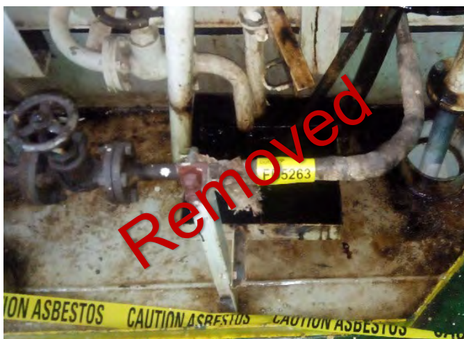
Photo 51 FD5263 4th Deck, Engine Room, Port, Primary Bilge Tank Steam Drain Line, Woven Rope (Chrysotile)
