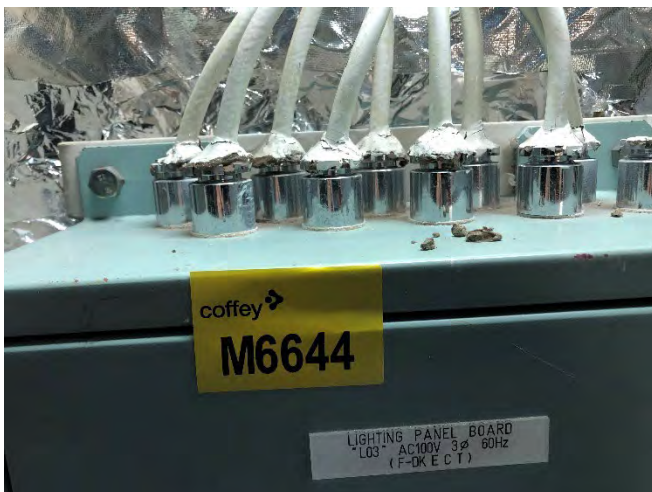
Photo 87 M6644 F Deck – Electrical Cable Trunk – On top of lighting panel board -Stbd Aft, Putty Mastic Material Debris (Chrysotile)
