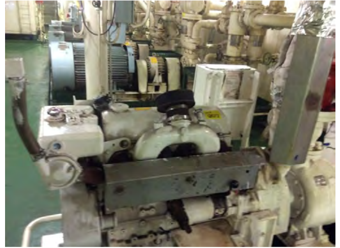
Photo 42 Q5373 Focsle store - aft -emergency fire generator Exhaust manifold Gasket
