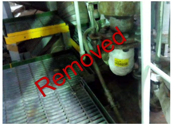
Photo 56 FD5238 2nd Deck, Engine Room, No.2 Boiler Drum Safety Valve, Forward, Woven Rope (Chrysotile)
