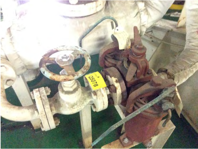
Photo 65 Q5078 4th Deck – Main Engine Room – Grease Extractor, Gasket (Chrysotile)
