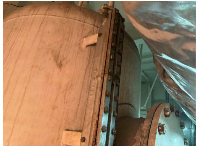
Photo 46 Q5324 A deck - incinerator room sludge tank gauge 2nd sight glass Gasket
