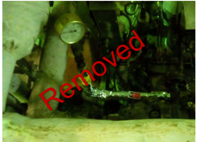
Photo 58 FD5240 2nd Deck, Engine Room, No.1 Boiler, No.1 Burner F.O. Gauge Line, Woven Rope (Chrysotile)
