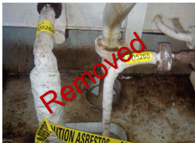
Photo 52 FD5264 4th Deck, Engine Room, Port, Primary Bilge Tank Steam Heat Supply, Woven Rope (Chrysotile) & Non-ACM Adhesive (White)
