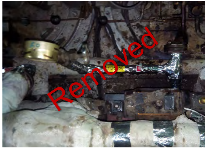
Photo 62 FD5250 2nd Deck, Engine Room, No.2 Boiler, No.1 Burner F.O. Supply Line, Woven Rope (Chrysotile)
