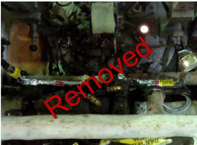
Photo 59 FD5241 2nd Deck, Engine Room, No.1 Boiler, No.1 Burner ATM, Steam Line, Woven Rope (Chrysotile)
