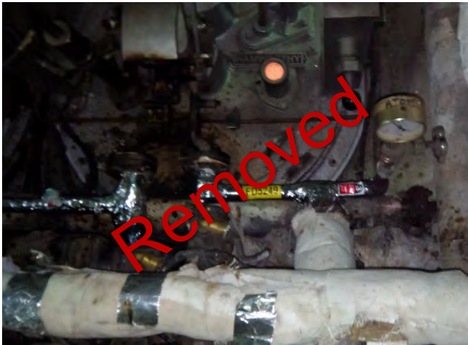
Photo 61 FD5249 2nd Deck, Engine Room, No.2 Boiler, No.1 Burner ATM, Steam Line, Woven Rope (Chrysotile)
