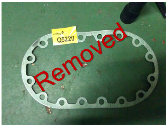
Photo 13 Q5220 2nd deck - IG room -Portside ships frame Loose Green oval Gasket
