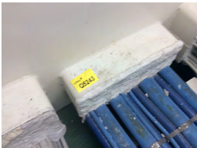
Photo 49 Q5243 F deck - cable locker Cable penetration insulation
