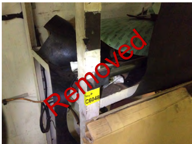
Photo 9 C6048 3rd deck - engine room workshop fwd - sheet Gasket packing shelf 2nd from top Grey sheet gasket debris on shelf
