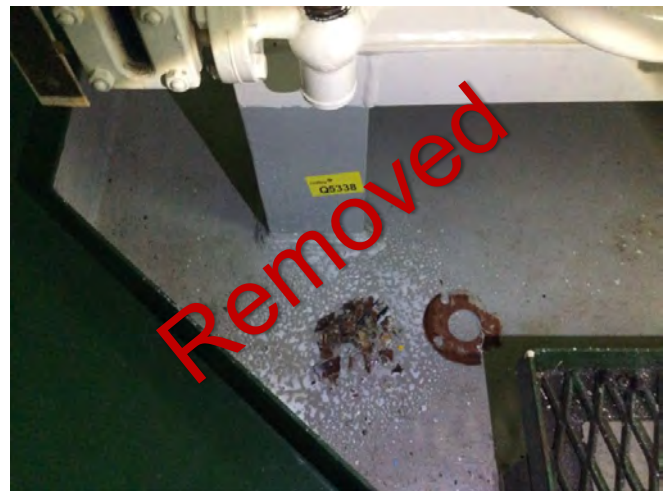
Photo 8 Q5338 3rd deck - steering flat - aft Winch hydraulic tank Gasket debris on ground
