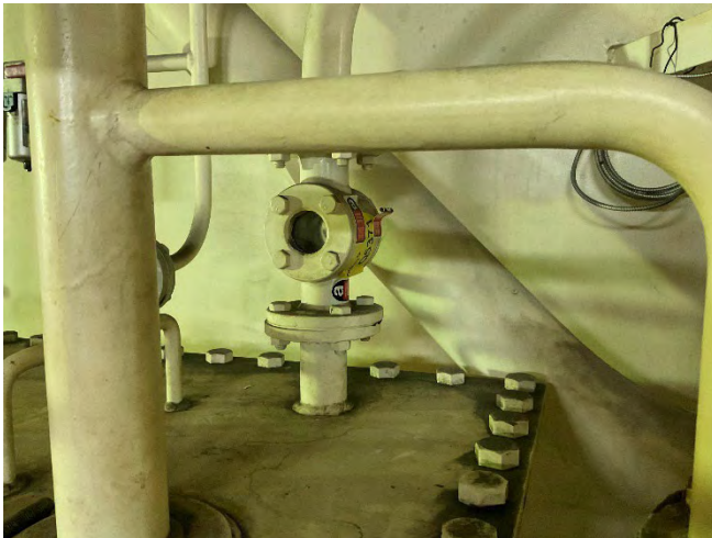
Photo 33 Q5371 Focsle Store -Starboard Aft - Hyd Oil Fuel Tank Return Glass Gasket to hyd oil tank return glass gasket
