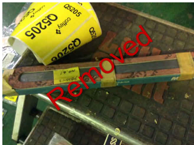
Photo 30 Q5204 2nd deck - 2sa -starboard side bulkhead German made sight glass Gasket brand unknown
