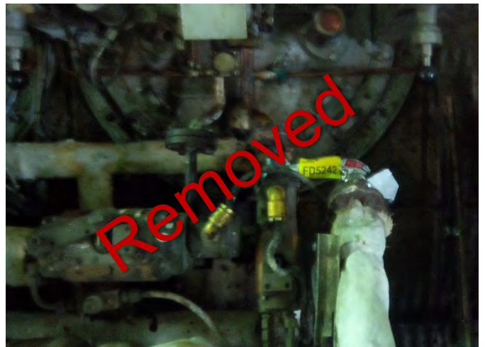
Photo 60 FD5242 2nd Deck, Engine Room, No.1 Boiler, No.2 Burner ATM, Steam Line, Woven Rope (Chrysotile)
