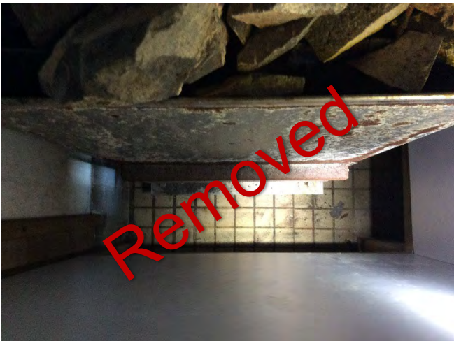
Photo 67 Q5052 2nd Deck, Sauna, Fibre Cement Debris (Chrysotile)
