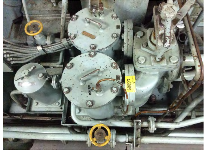
Photo 66 Q5089 3rd Deck – Generator No.1 Room – Gasket to L.O, Filter Casing, Gasket (Chrysotile)
