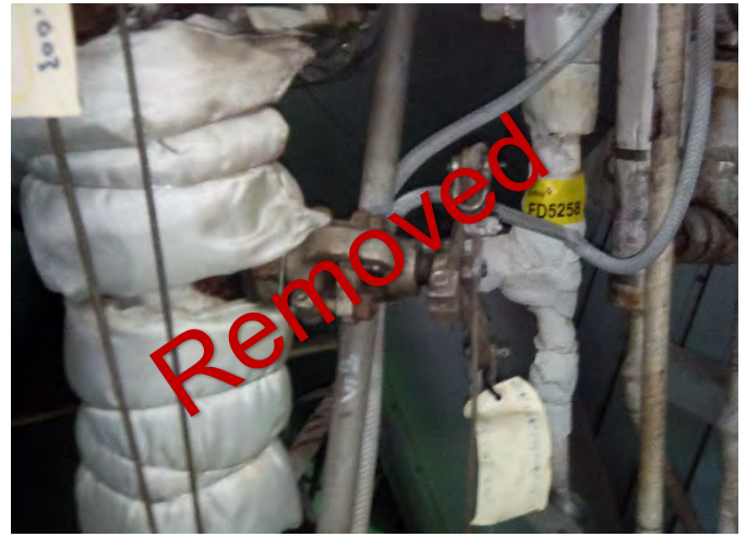
Photo 54 FD5258 Boiler Gauge Glass Level, Engine Room, No.2 Boiler Level Transmitter (Port), Woven Rope (Chrysotile) & Non-ACM White Adhesive.
