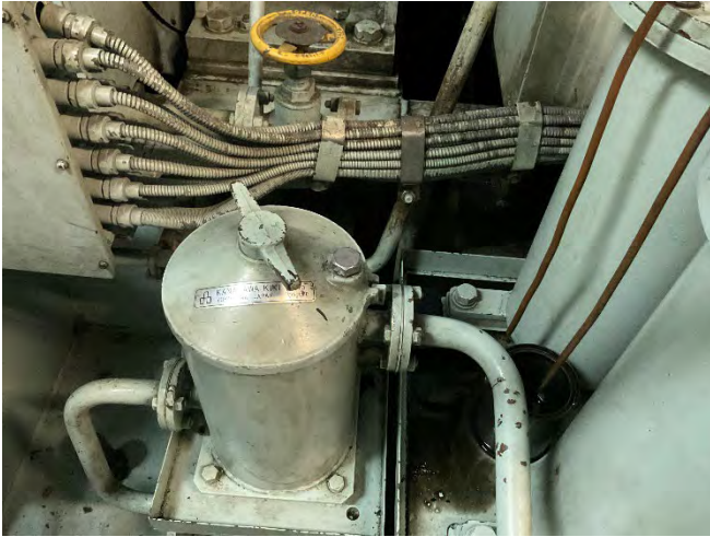
Photo 93 ZA21825 3rd Deck Lube oil system to Generator 2 Gasket Adjacent walkway Port Side (Chrysotile)
