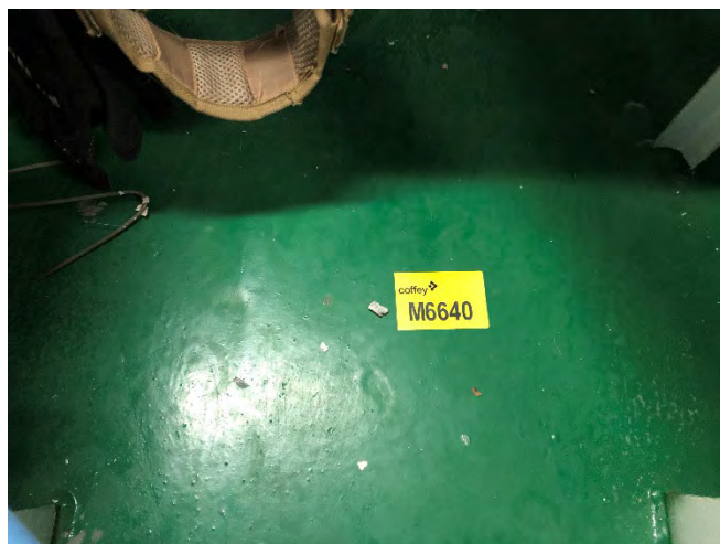
Photo 86 M6640 F Deck – Electrical Cable Locker – Stbd Fwd - Penetration Material Debris (Chrysotile)
