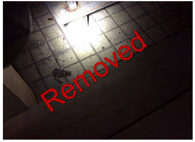
Photo 68 Q5052 2nd Deck, Sauna, Fibre Cement Debris (Chrysotile)
