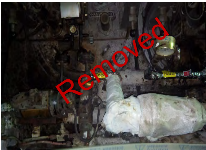
Photo 63 FD5251 2nd Deck, Engine Room, No.2 Boiler, No.2 Burner ATM, Steam Line, Woven Rope (Chrysotile)
